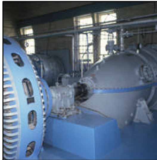
One of the pumps at the Utah Lake Pumping Plant as seen in 1995.
