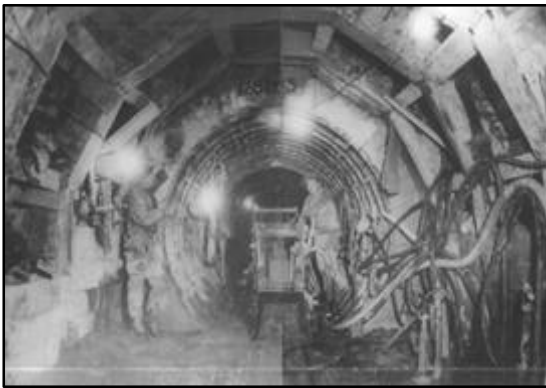
The Deer Creek Aqueduct (Salt Lake Aqueduct) Alpine Tunnel work during the summer of 1939.
