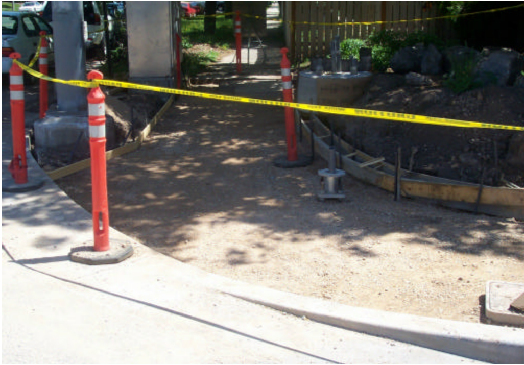
Does this look safe? How would a person with a visual disability navigate this construction site?
