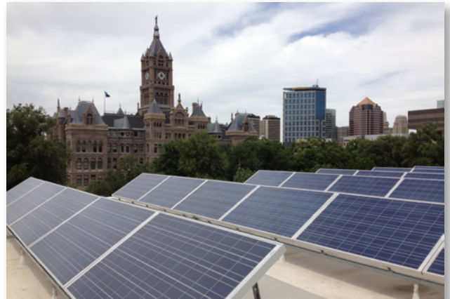
View from the Public Safety Building rooftop solar installation.
