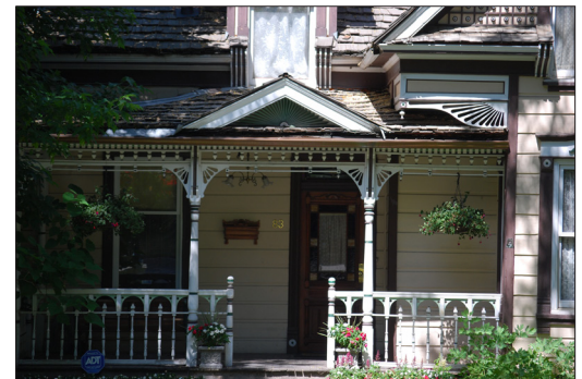
Repair original elements of the porch and consider reinstating original features which have been lost.
