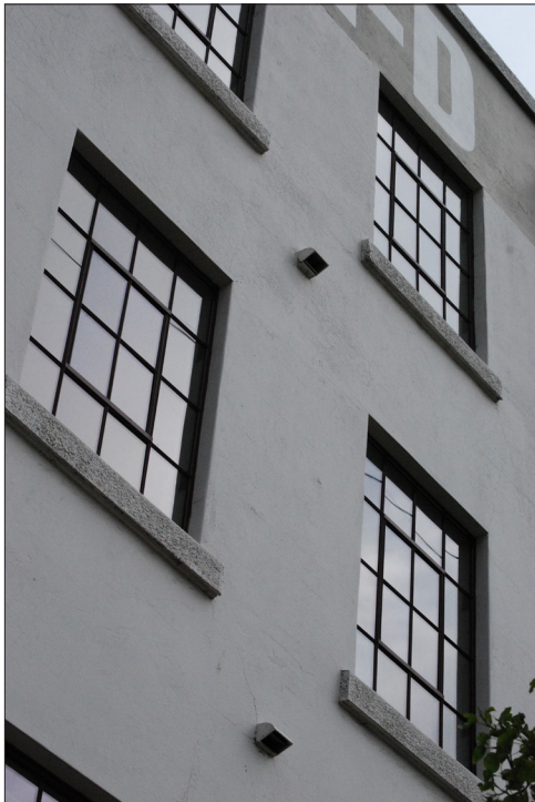
Rehabilitation of the building here involved retaining, repairing and upgrading the original steel framed windows.
