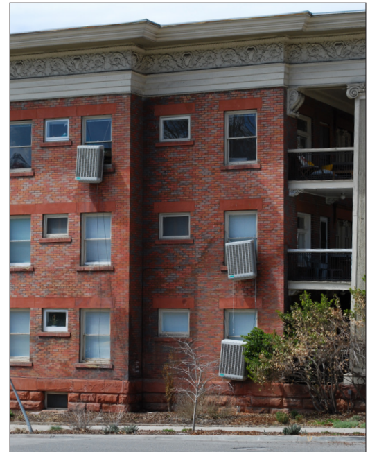
Coordination of air conditioning equipment can avoid sporadic placement on important street facades.
