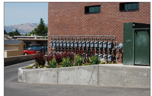
Screening of utility service meters in this instance will rely on maturing landscaping and subsequent maintenance.
