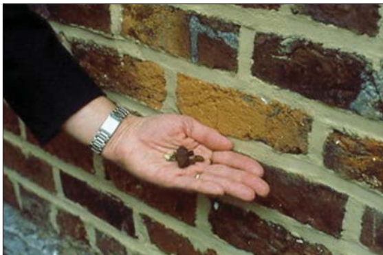
Hard impermeable modern mortars force moisture through the more permeable brick and allow mechanical stresses to be relieved through the softer brick which may lead to cracking, spalling and erosion. Here, new mortar fails to match the original.
