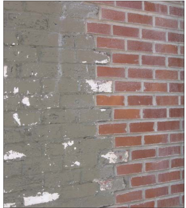
Painting brick changes the character of a building.
