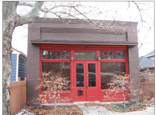
Woodwork is a character-defining feature of this storefront at 361 N. Main Street.
