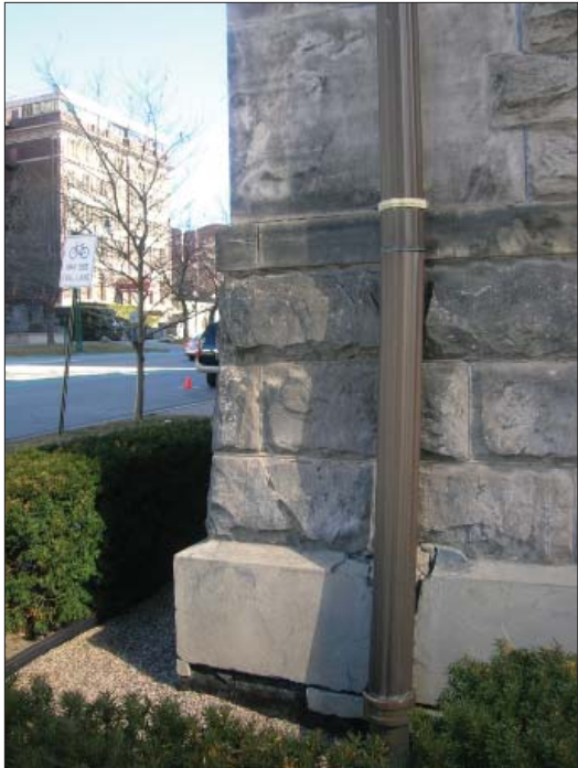
Moisture, wind-borne grit and pollutants can affect all types of foundation materials.
