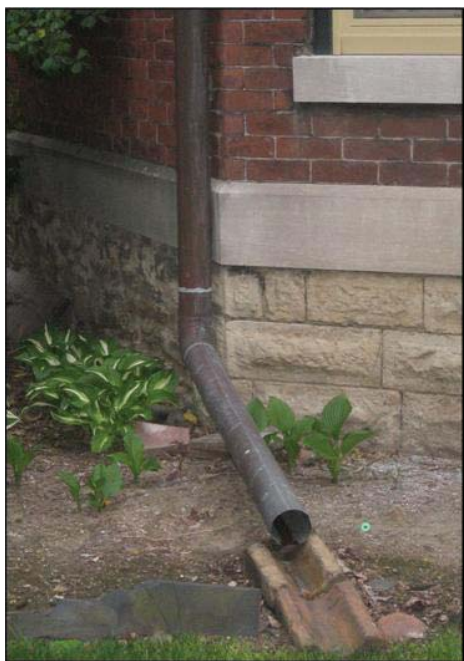
An appropriate downspout and splash block.
