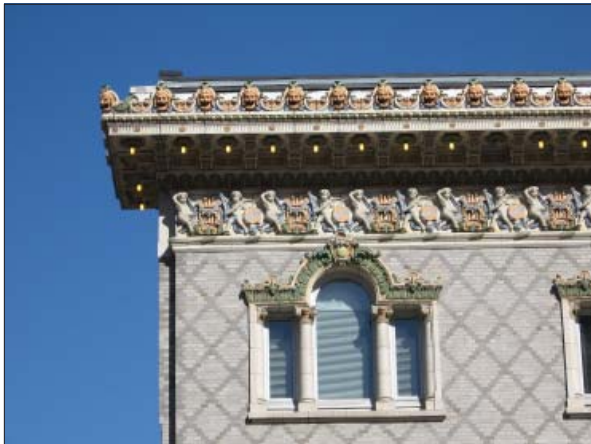
Architectural details of the Capitol Theatre include an ornate cornice and decorative window hoods and surrounds.
