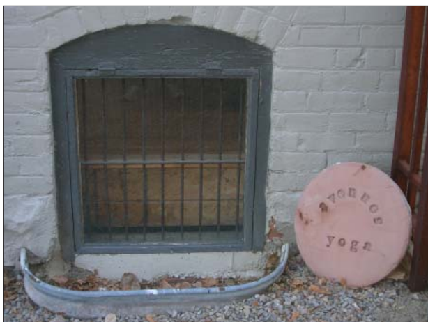
Installing security bars on the inside of windows is a solution that accommodates both design and security considerations.
