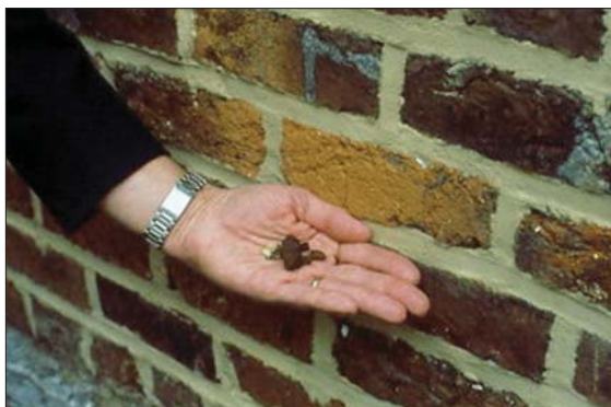
Hard impermeable modern mortars force moisture through the more permeable brick and allow mechanical stresses to be relieved through the softer brick which may lead to cracking, spalling and erosion. Here, new mortar fails to match the original.
