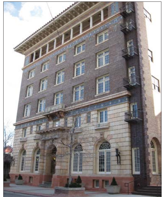
The appearance and integrity of original masonry can be successfully maintained through appropriate repair. Commercial Club Building, 32 Exchange Place.
