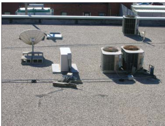
This low-profile mechanical equipment is situated in an inconspicuous area on top of the building.
