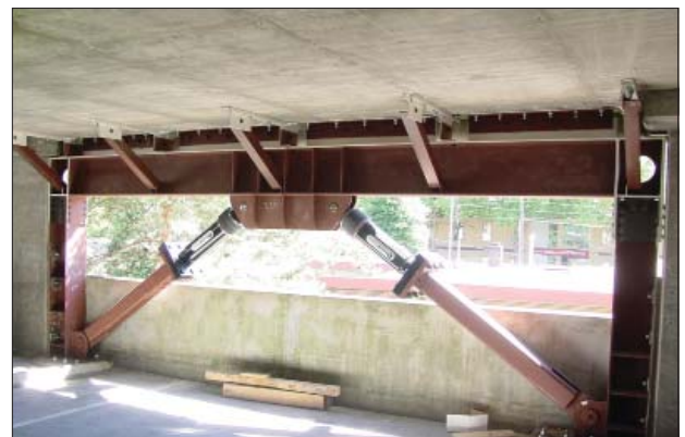
Seismic retrofitting can include adding steel frames and dampers in basement and parking areas of commercial buildings.
