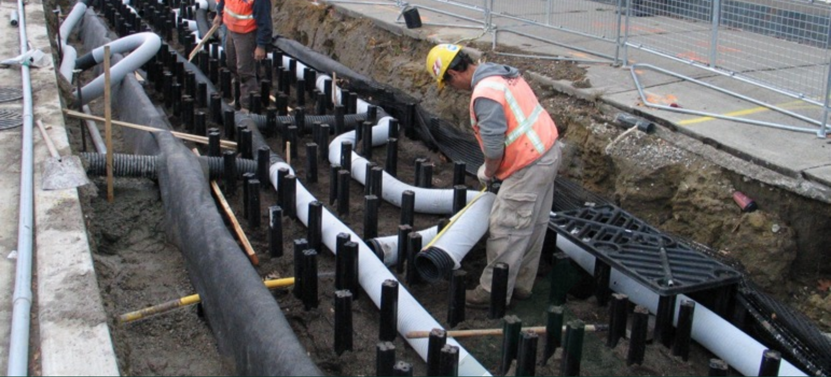
Suspended pavement systems allow roots to thrive, growing large, healthy trees, while also storing overflow stormwater. Photo above shows a Silva Cell™ System being installed in Toronto, Canada 2010 (Deeproot.com)
