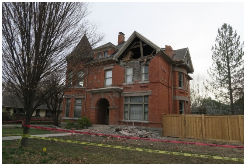
Figure 2: Photograph of damage to Sears Mansion following March 2021 earthquake.
