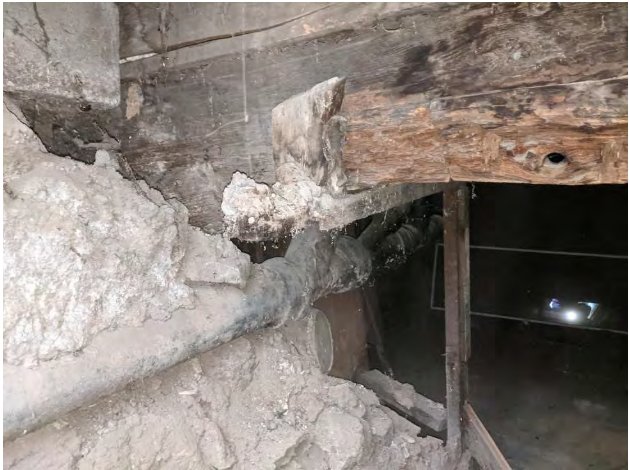
Entrance to basement from inside the house. Again the wood perimeter joist is buried in earth.
