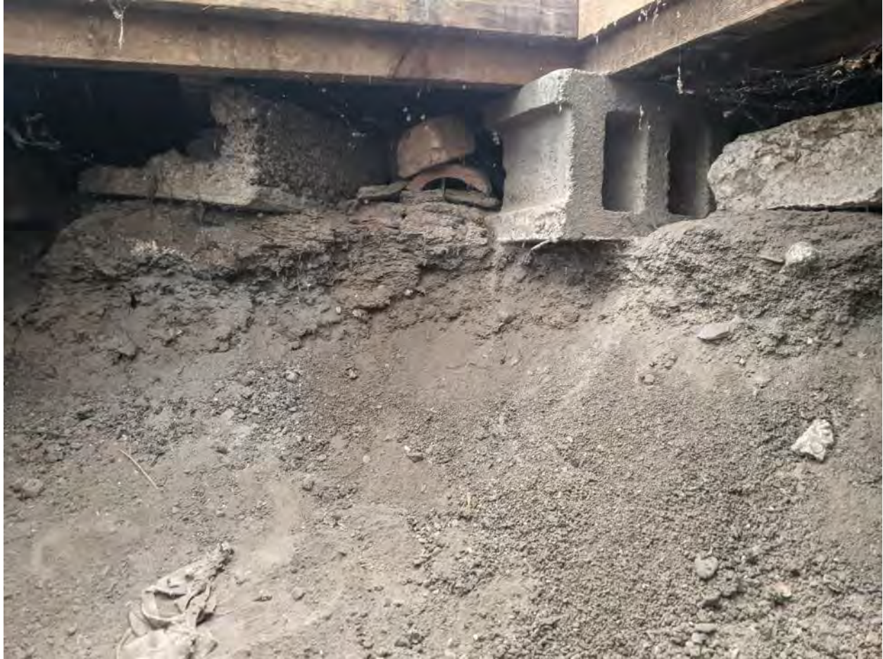
Typical shoring attempt.
