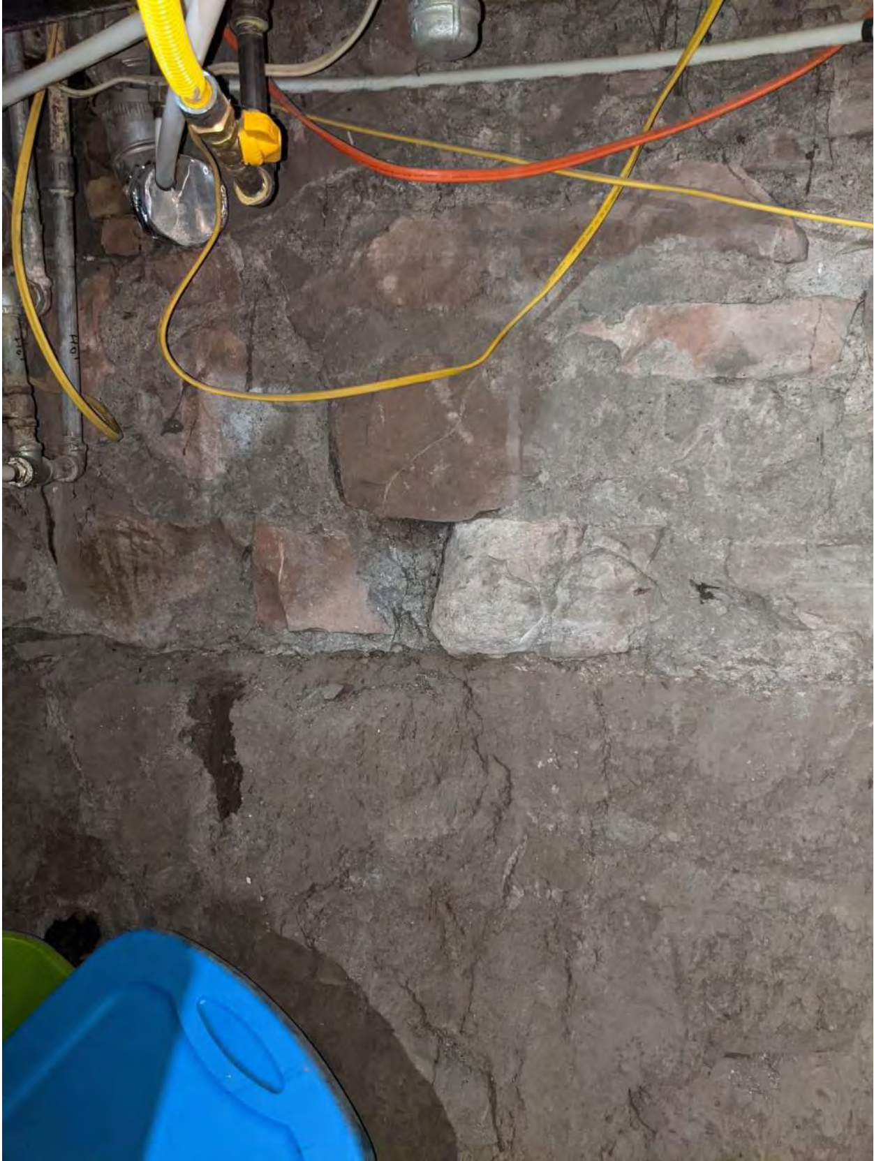
Earth beginning to undercut the foundation wall.
