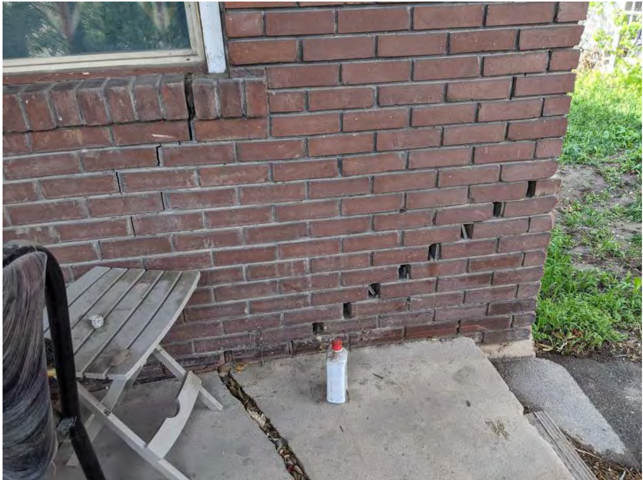
Exterior North West corner. Foundation is rolling outward.
