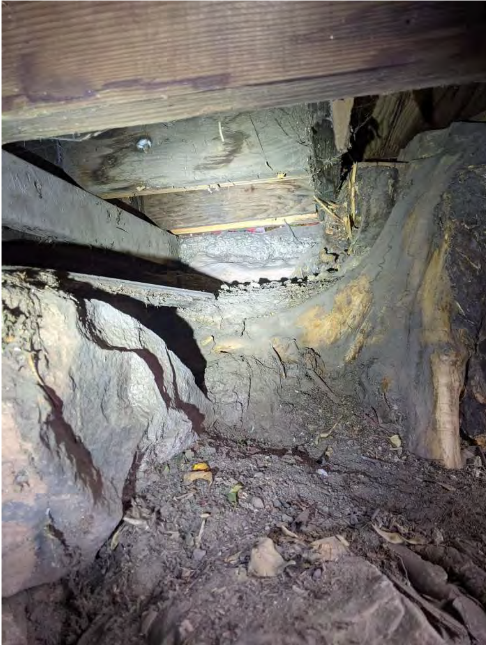
South East corner of foundation sitting on earth and previously compromised by a tree. Temporary concrete shoring visible.
