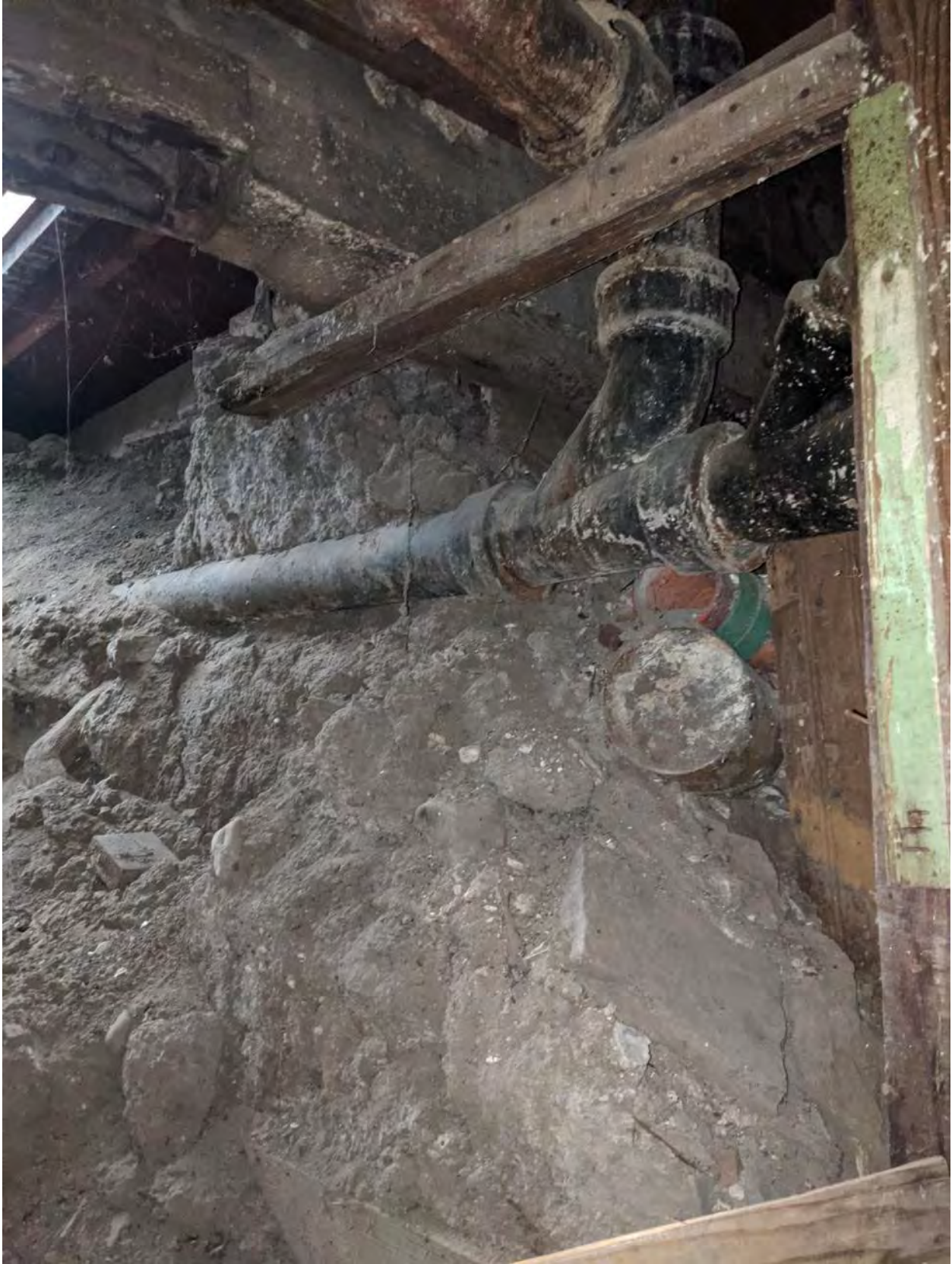
South West foundation bearing on collapsing earth.
