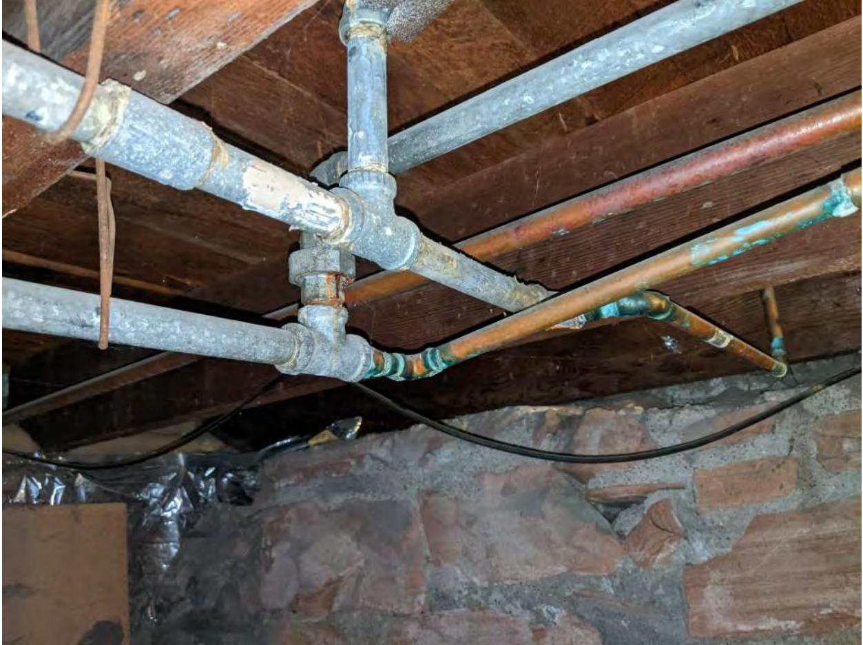
Again a mix of water supply materials installed without proper unions. Galvanic decay present.
