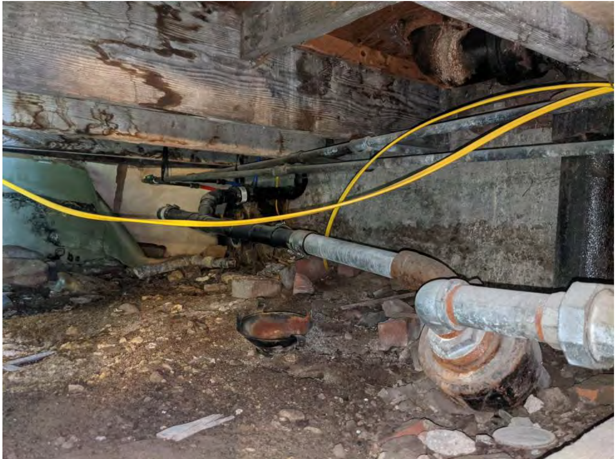
Typical plumbing with repair work.
