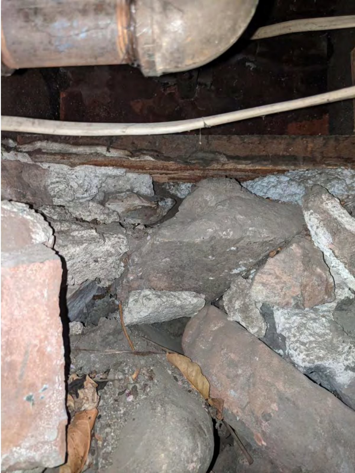
East foundation collapse
