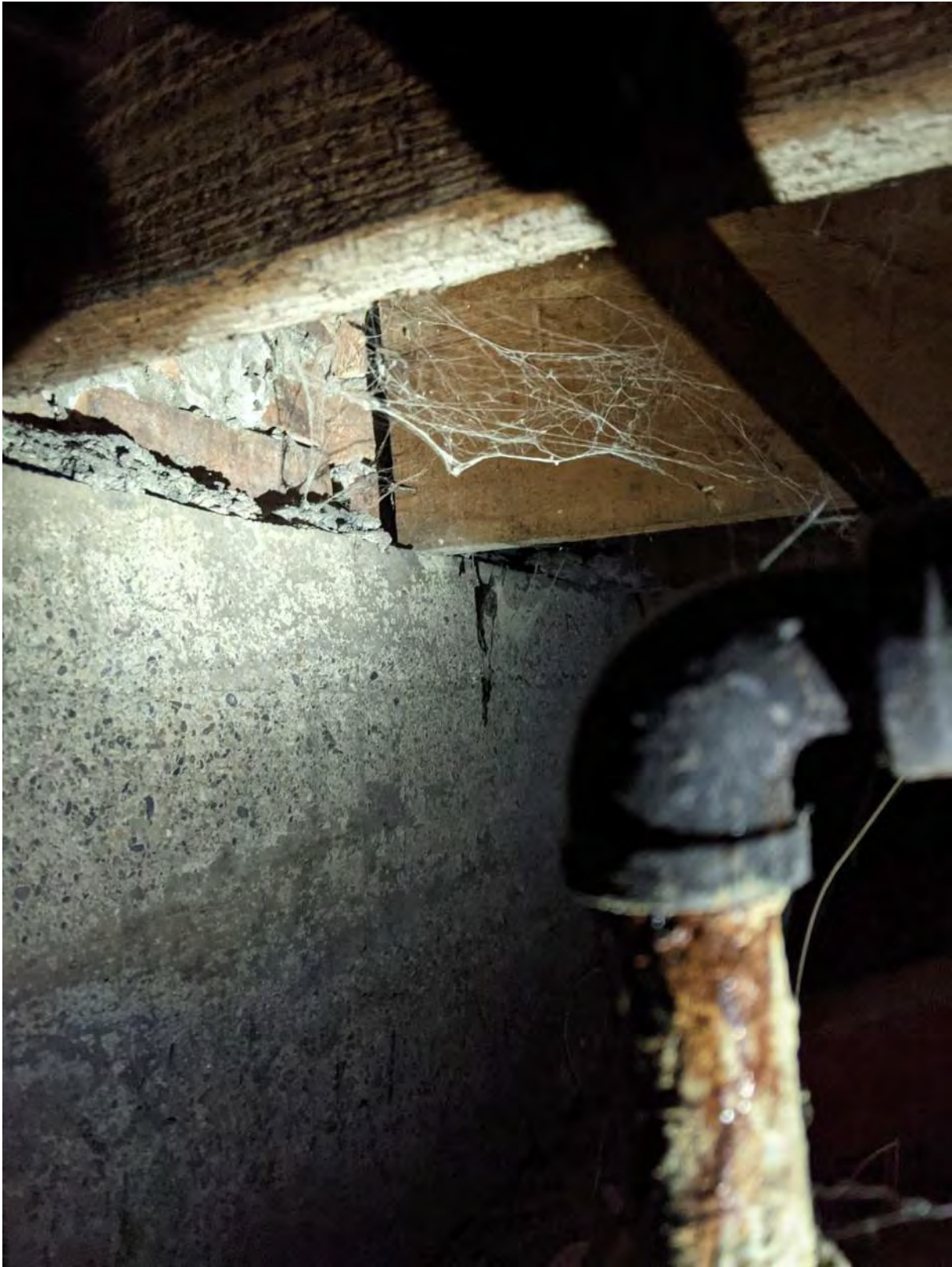
Floor joist coming off of foundation. Typical along western foundation length.
