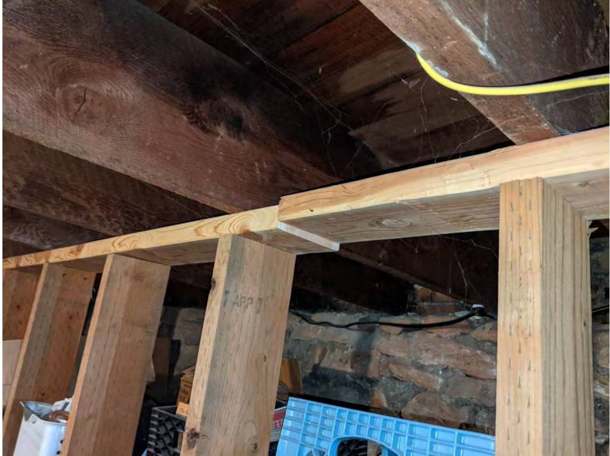
Improperly spliced top plate. A staggered double top and bottom plate would likely be required.
