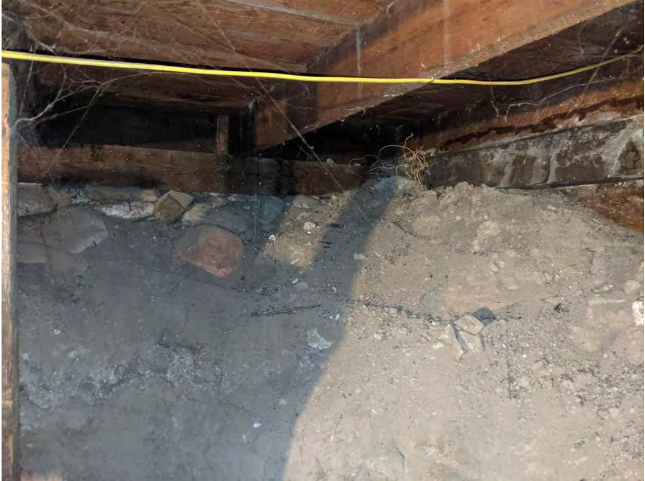
North West corner of foundation. Note 2x6 floor joists 24" on center, typical of entire floor assembly.
