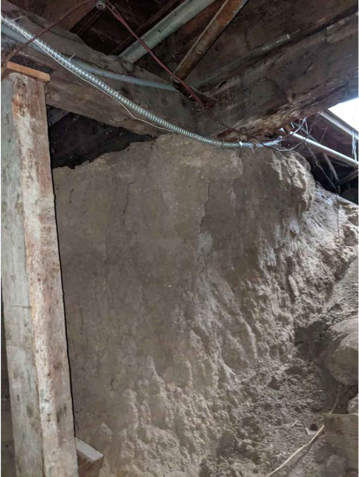
South East foundation bearing on earth that's caving in. This is also the basement access.
