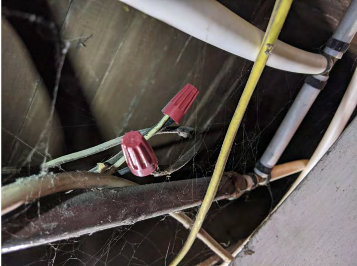
Romex tied into old knob and tube wiring.
