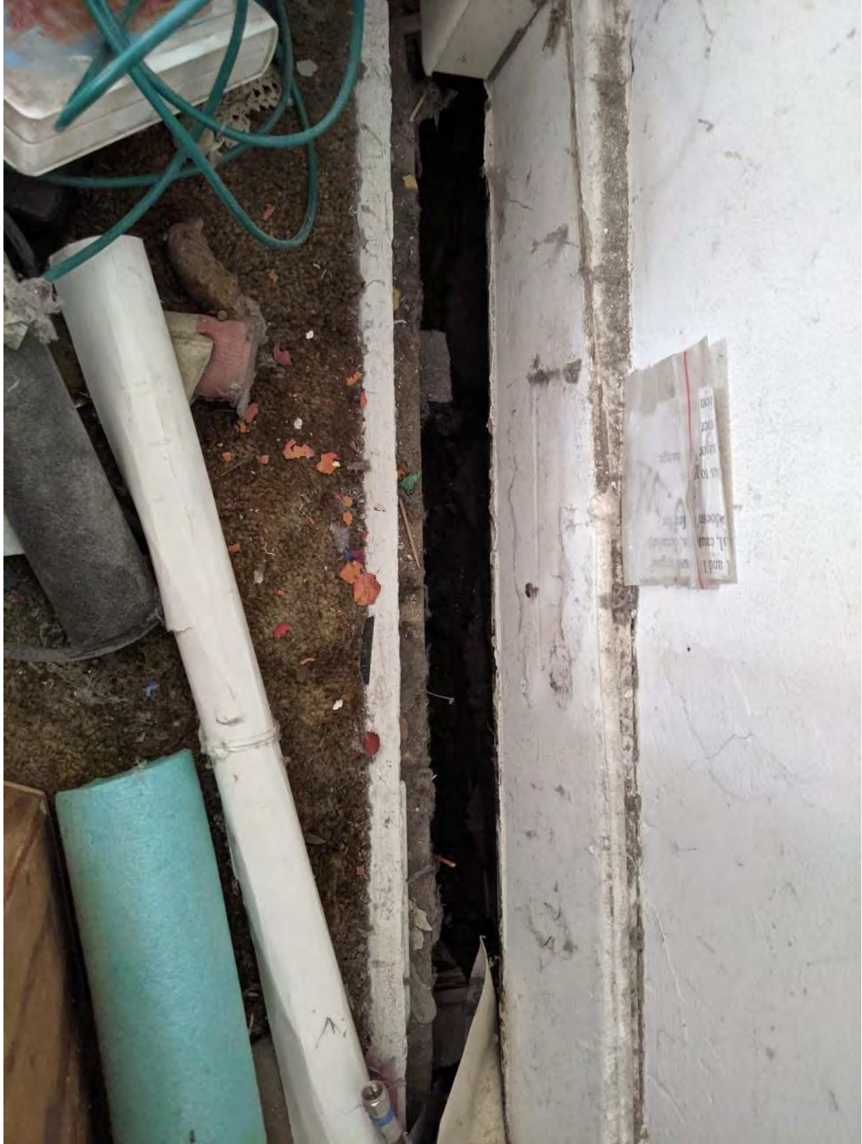
Western wall has pulled away from floor assembly for nearly the entire length of the house.
