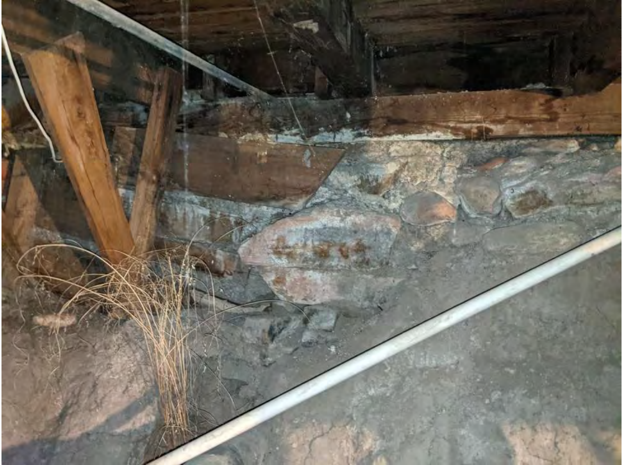
Western foundation collapse. Poured concrete shoring present.
