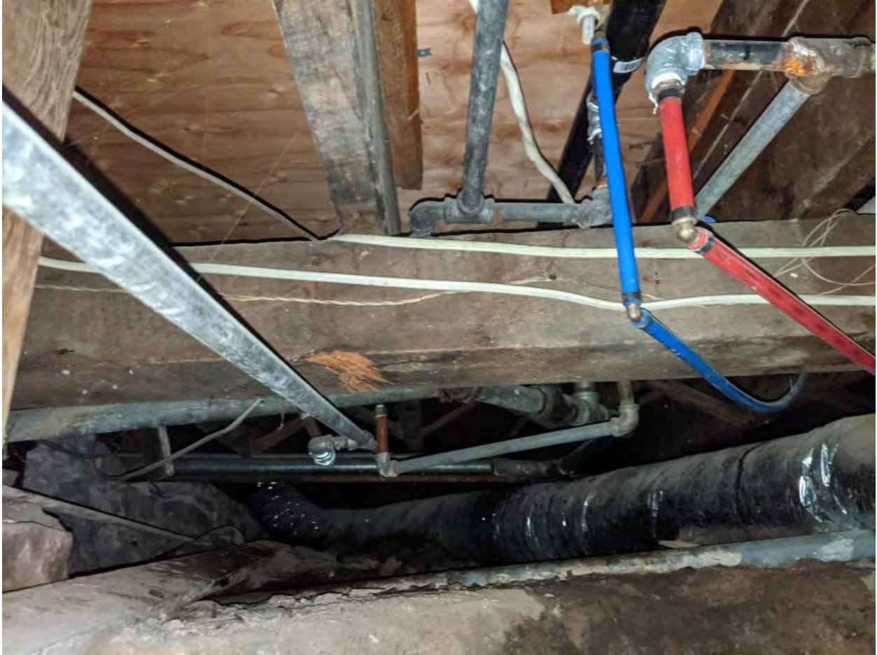
Typical plumbing condition. PEX, copper, galvanized and black pipe in non code compliant installation.
