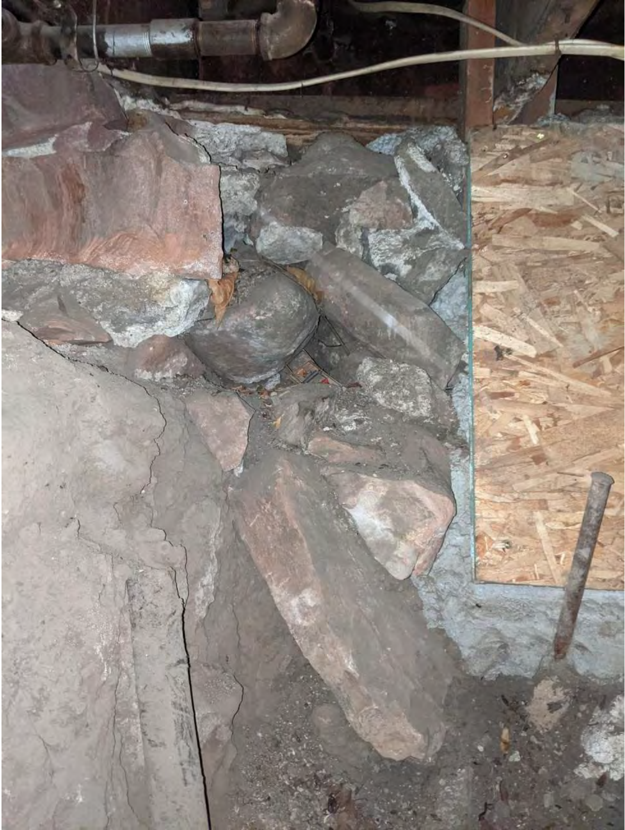
East foundation collapse with more temporary concrete shoring.
