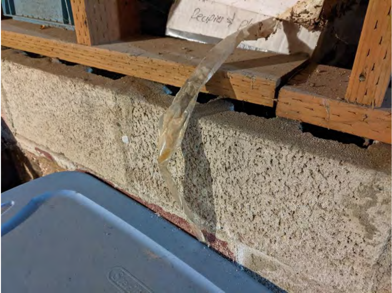
Improperly spliced base plate. No double plate. Hollow CMU's. No reinforcement.
