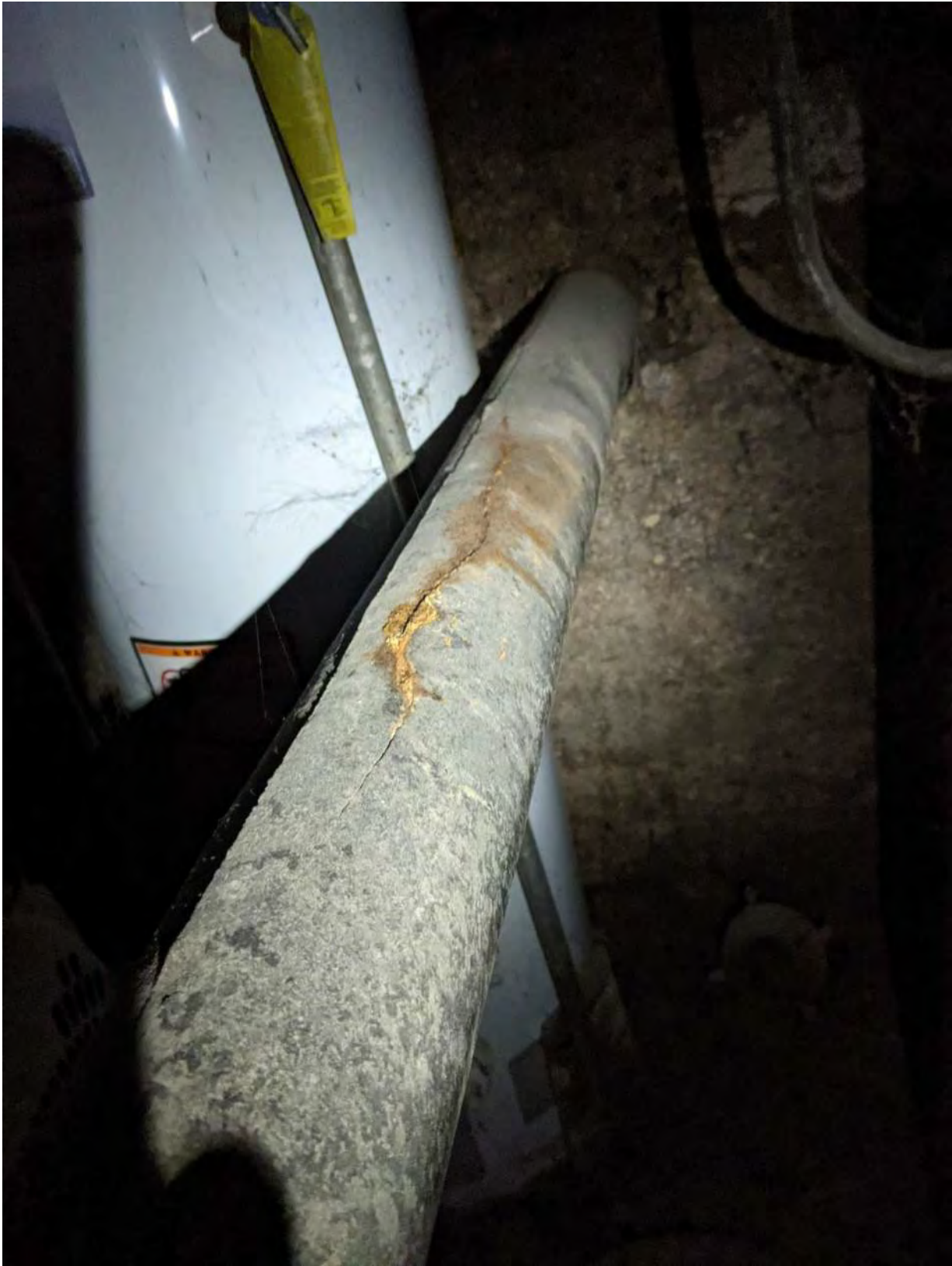
Cracked sewer line. Typical of condition.
