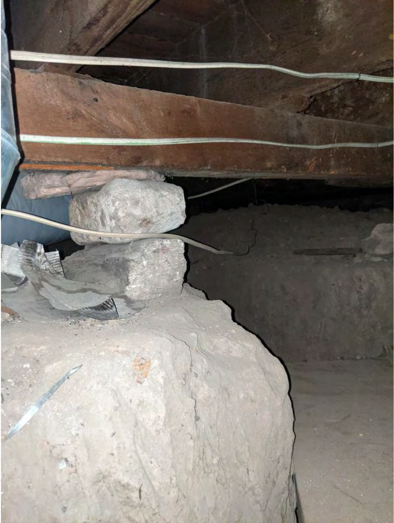
Unreinforced span support (typical)
