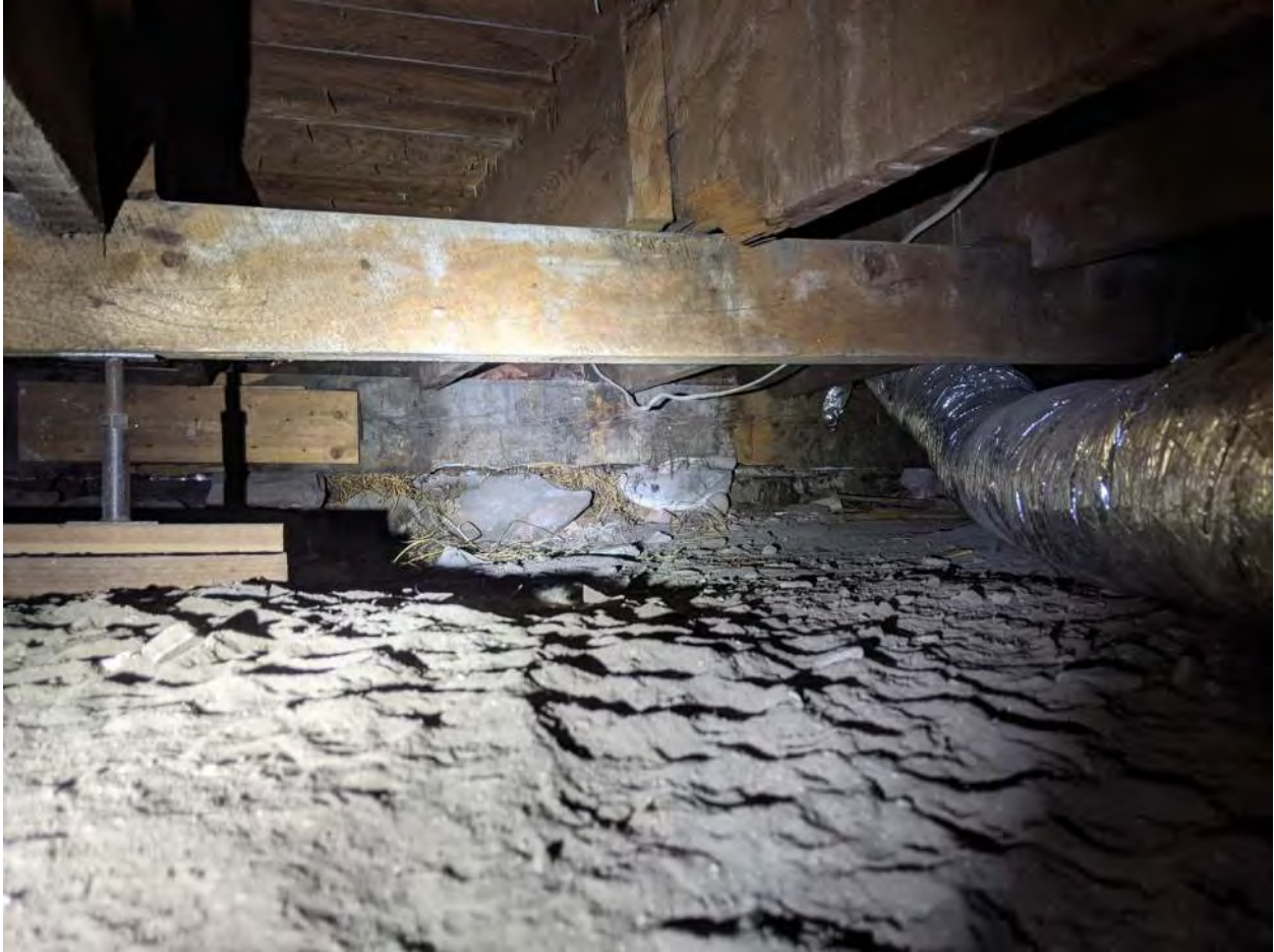
Western foundation joist bearing on earth and loose sandstone rock.
