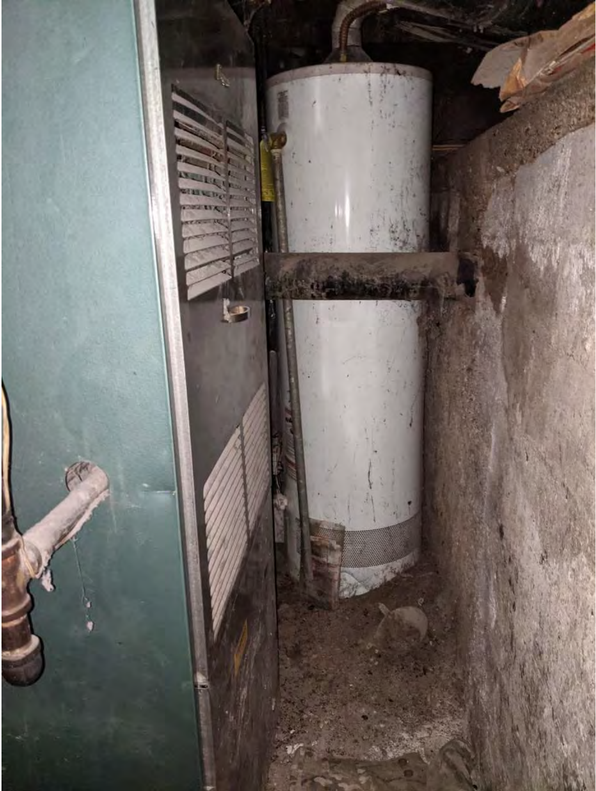
Rain water as well as waste water back flows into this area.
