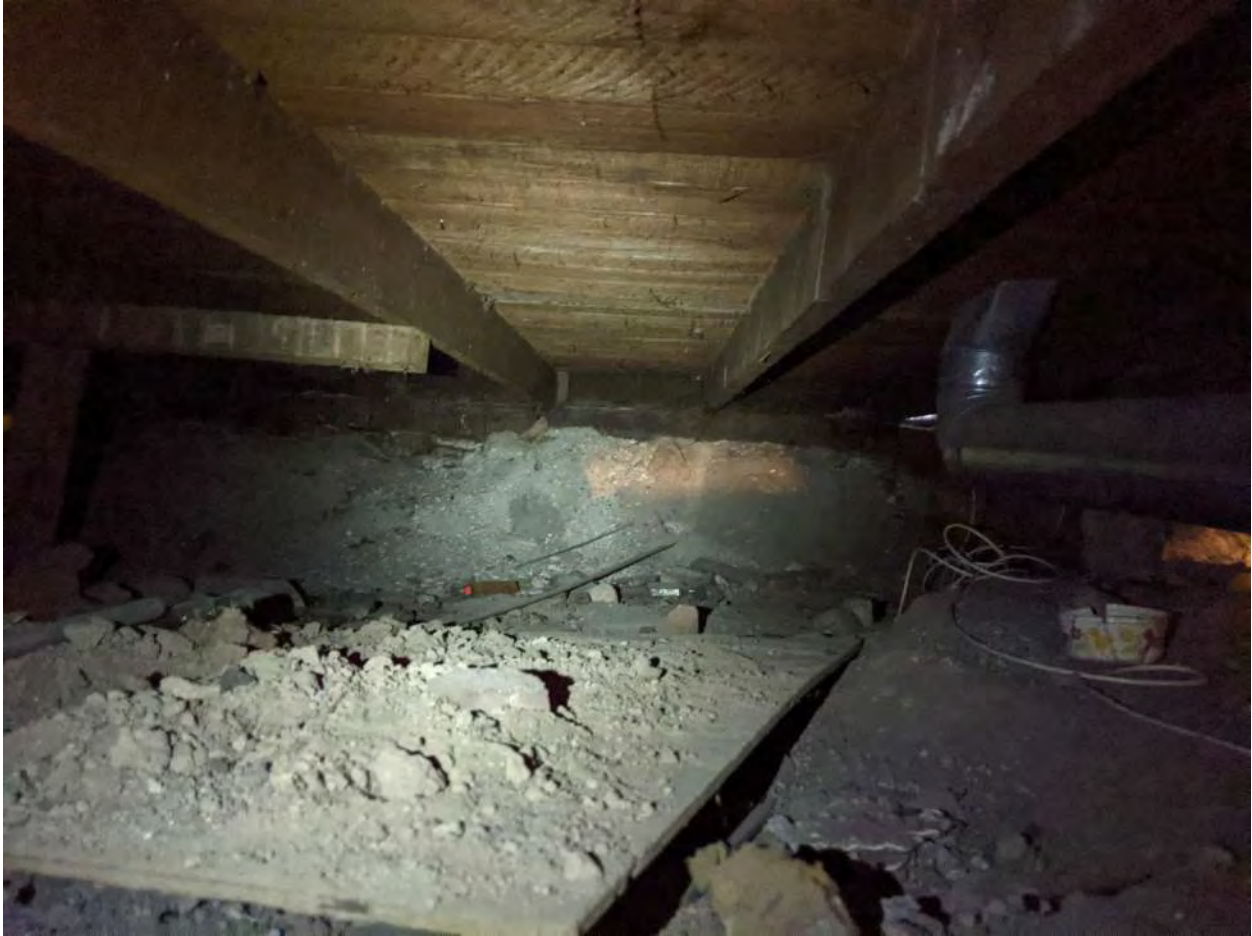
Eastern foundation joist bearing in earth. Again 2x6 floor joists 24" on center. Typically these would be 2x8's or 2x10's 16" on center.
