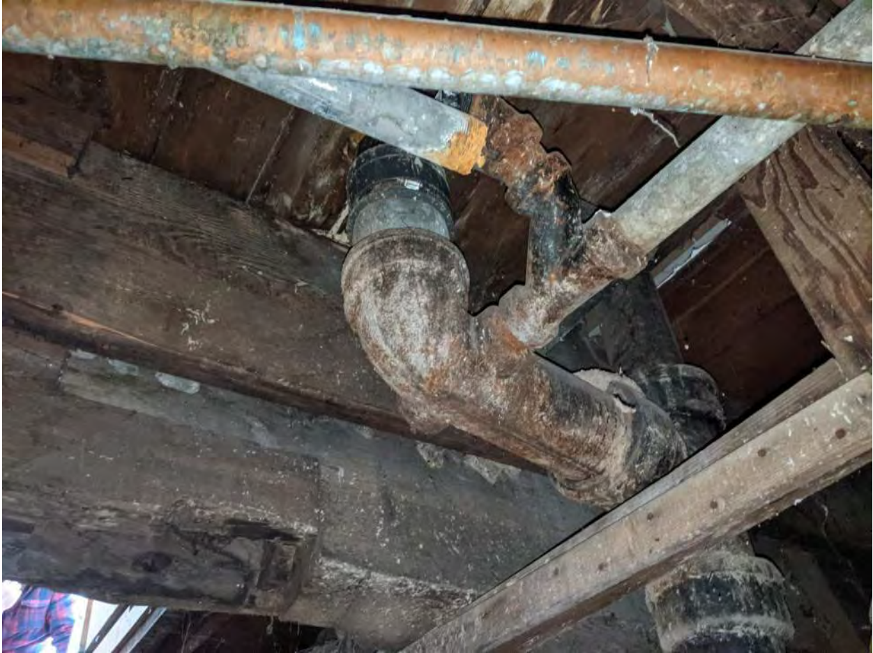
Typical cast iron plumbing.
