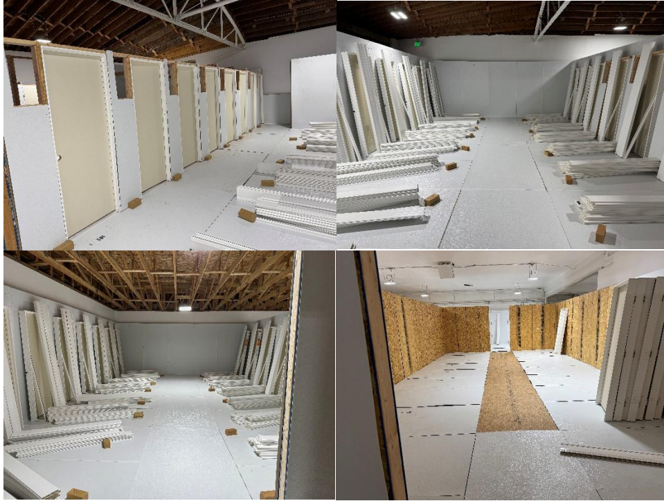
Pictures show in progress construction of individual rooms. 6 foot removable modular fencing is secured between each room and can be removed or added depending on the preference of the customer expanding space.
