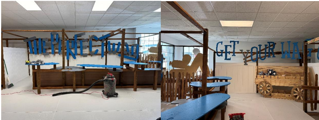
The showroom is elevated to demonstrate the enclosed build of the rest of the building both kennels, hallways, and play yards. Walls and flooring are made of vinyl or FRP vinyl.
