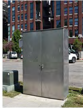
S12. Electrical Large Box
