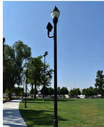
S3. Single Light Pole Ornate with Solar Panel
