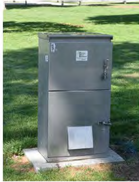
S11. Electrical Box
