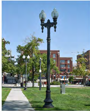
S5. Double Light Pole
