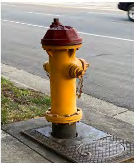
S29. Fire Hydrant
