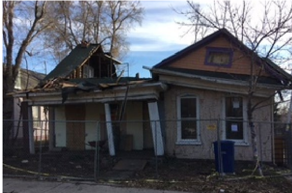
Figure 5 – Contributing house in the Avenues Local Historic District was severely damaged in 2017 after interior demolition resulted in the destabilization of the structure.
