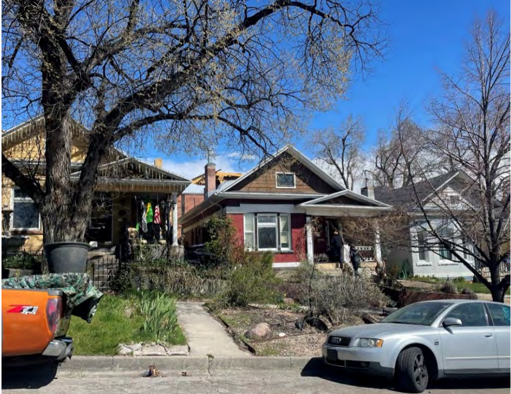
Subject property - under construction tree platform visible to the rear of the chimney
