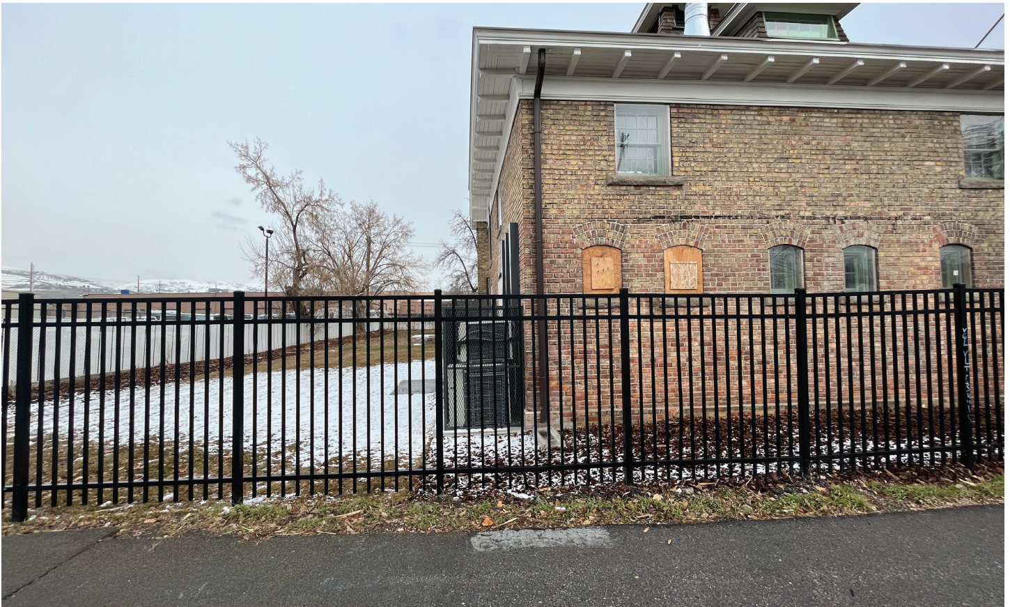
View 9 Looking E directly at HVAC units and cages at rear of Carriage House, from trail
