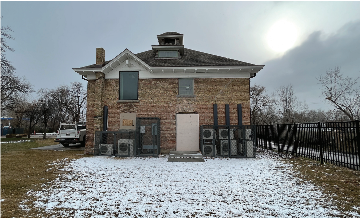
View 3 Looking S from rear of property looking directly at condensers and cages
