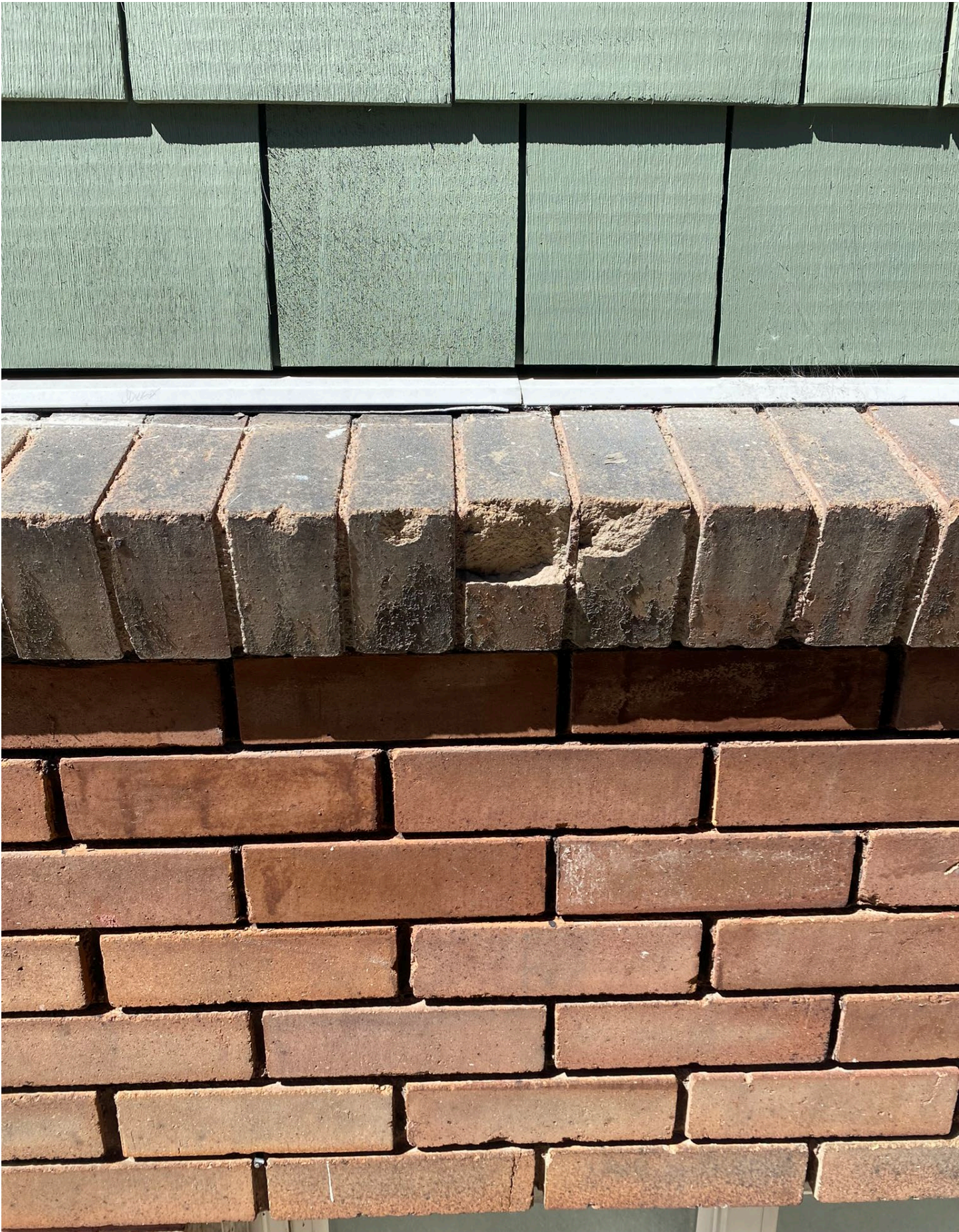
Damaged brick that needs repair
