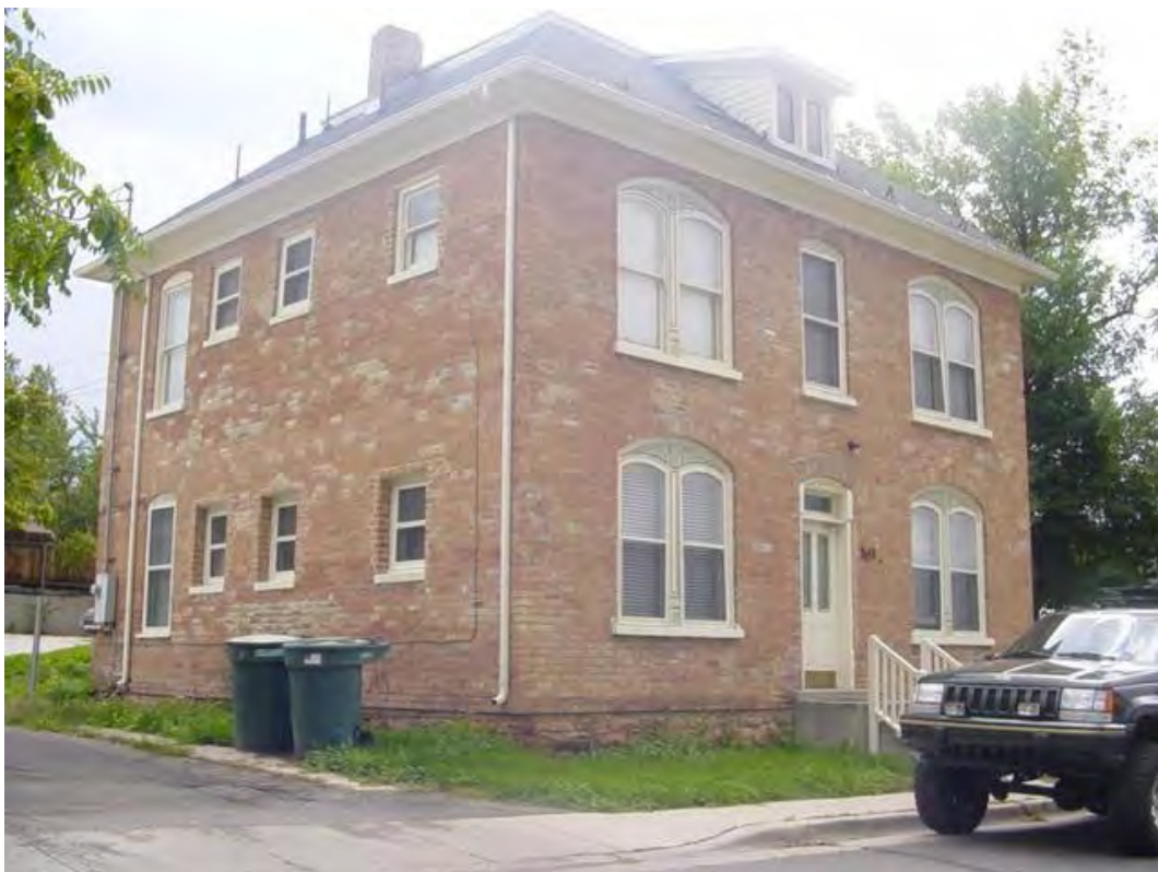
Subject property, c. 1995. The brick and sandstone foundation are unpainted. Spalling and repairs to mortar are also visible.
