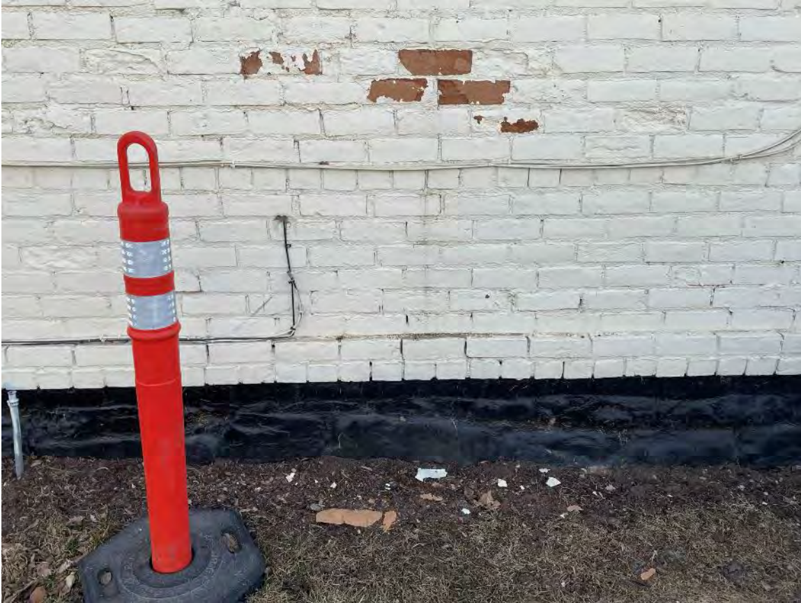
North façade, February 2022. Recent spalling of the brick is visible.
