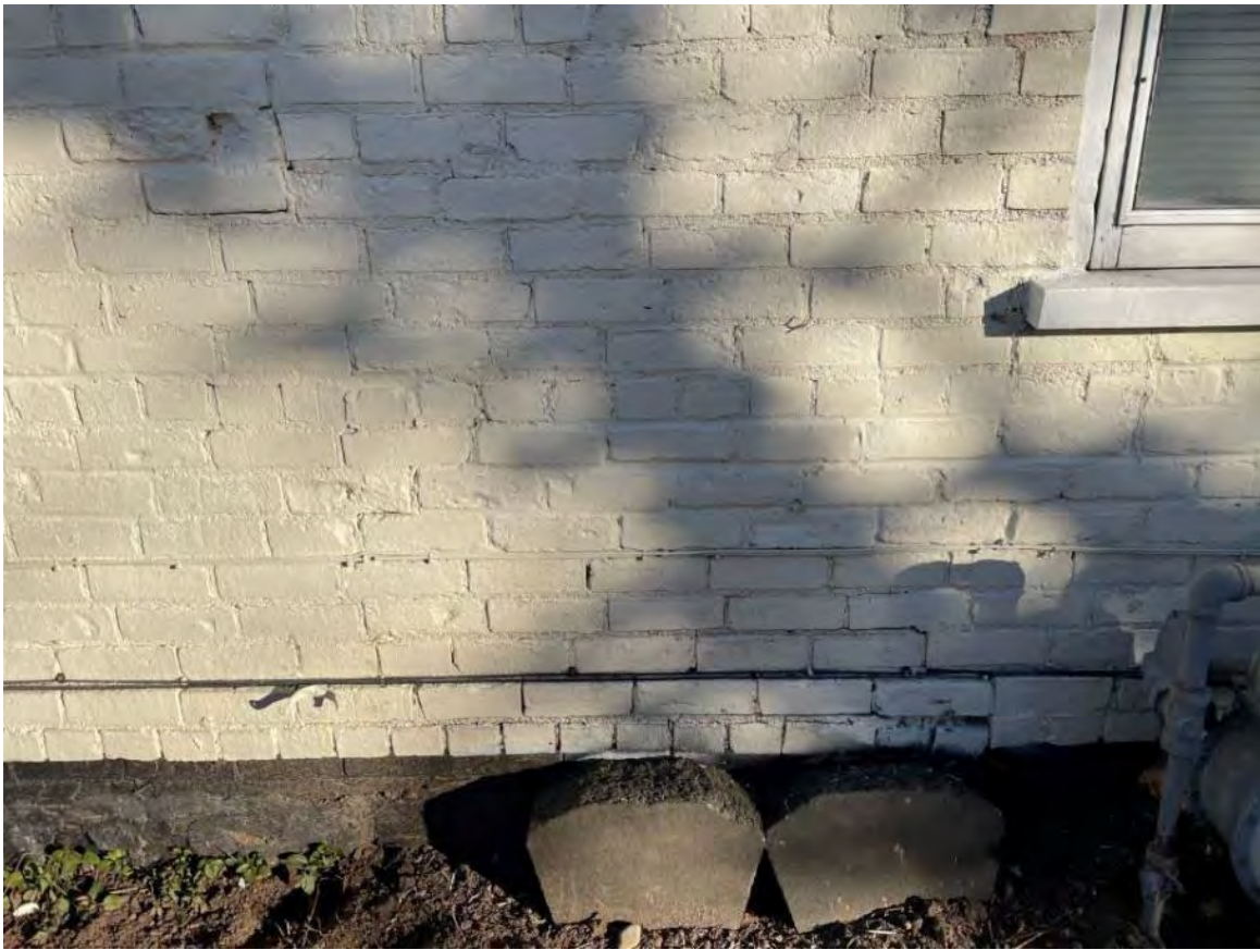
South façade, January 2022. Previous spalling and mortar repairs are visible.
