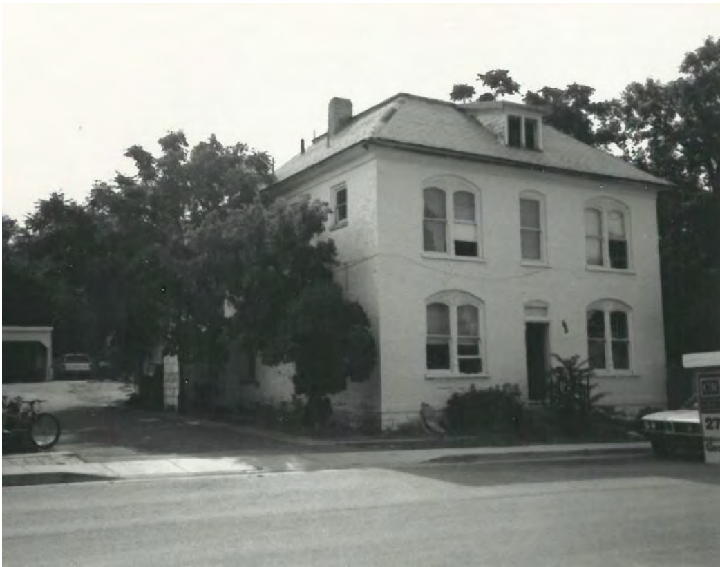
Architectural survey photo, c. 1980. The brick and sandstone foundation are both painted.
