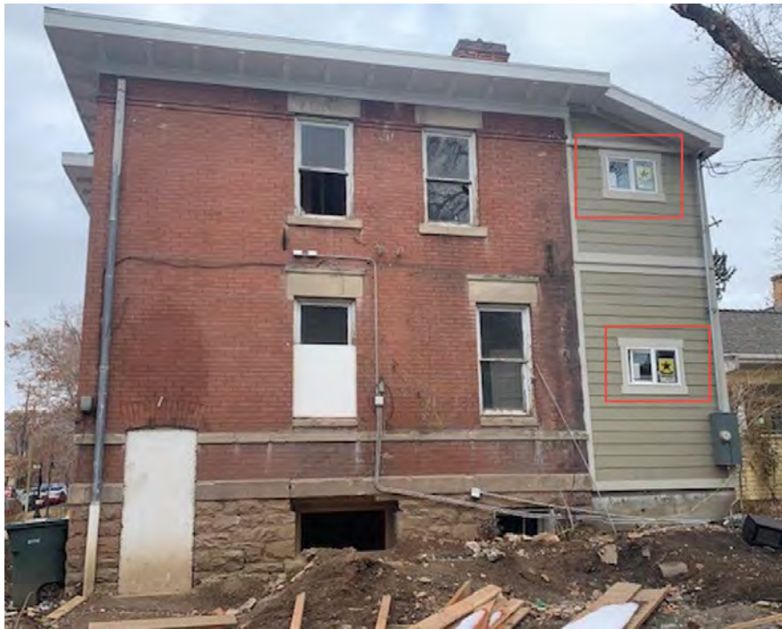
Installation of Incorrect Windows on the Southern
