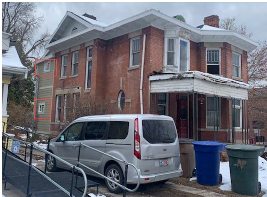
Installation of Incorrect Windows on the Eastern Elevation
