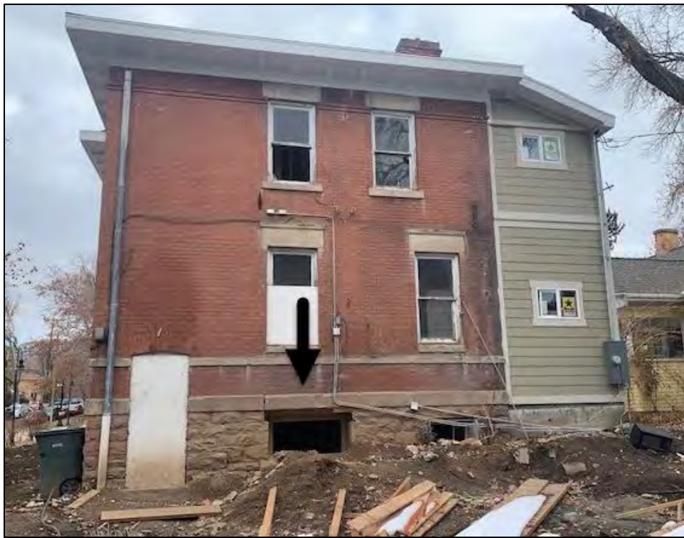
Post Enforcement Photo of South Elevation
