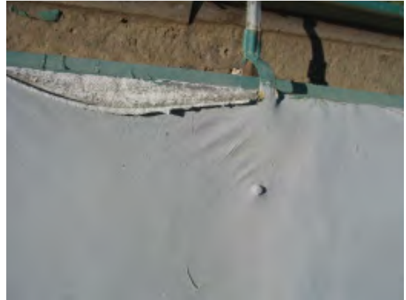
Figure IV-12. A detail of the edge of the porch roof showing the coating over the soldered metal peeling away.
