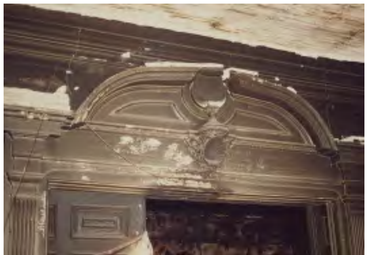
Figure III-51 (top right). A detail of the woodwork following the 1979 fire.
