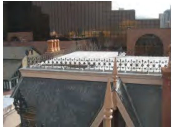
Figure IV-25 (above). A view of the east wing roof showing ponding water at the west edge.
