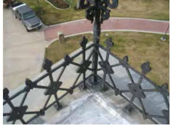
Figure IV-24. A detail of the southwest corner of the west wing roof, showing the uncoated metal roof outside the perimeter of the cresting, and a coating applied to the field inside the cresting.
