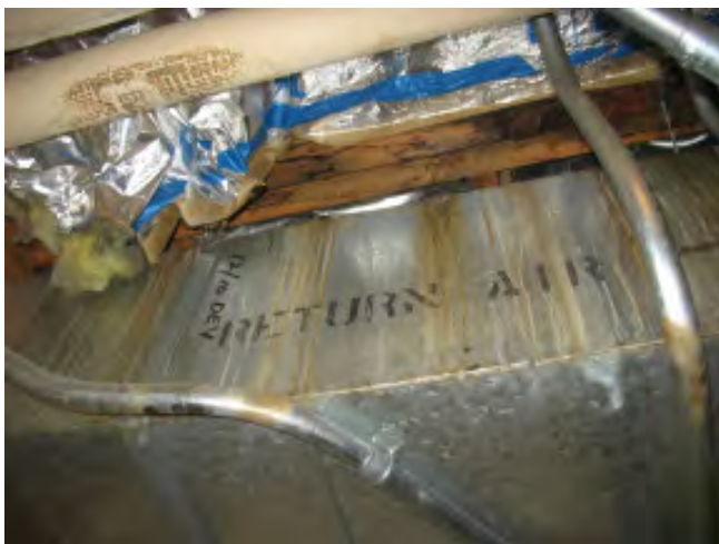
Figure IV-27. Staining due to roof leaks in the mechanical room under the east wing roof.
