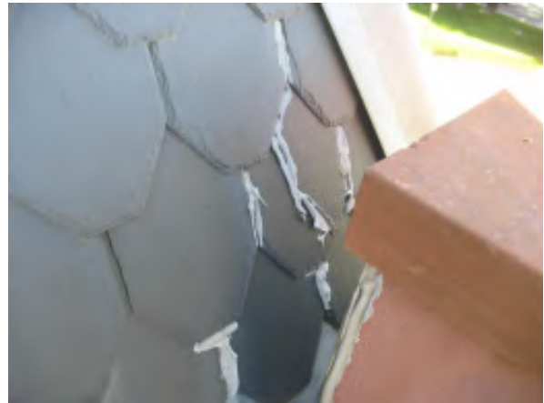
Figure IV-23. A section of roof slates on the east wing with sealant applied to the slate perimeters.
