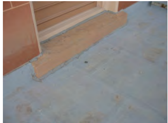
Figure IV-13 (above). A sandstone sill which interrupts the upturned leg of the metal roofing.
