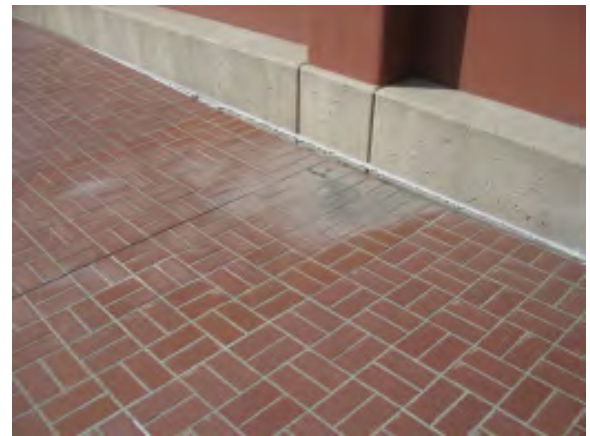
Figure IV-39. An area of subsidence in the patio slab. Note the level of the sealant installed at the original patio level, and the staining caused by ponding water
