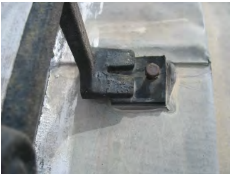
Figure IV-28. A detail of the supporting foot of the metal cresting which has slipped out of position.
