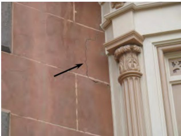
Figure IV-5. A detail of the crack at the location of the lintel bearing at the Drawing Room south bay window.
