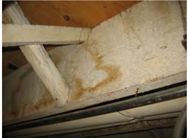
Figure III-31. Original joists and cross bracing in the east wing. Note the new plywood floor above.
