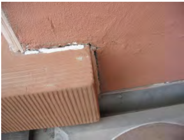
Figure IV-16. A detail of a window sill with an open breach where it meets the stucco wall.
