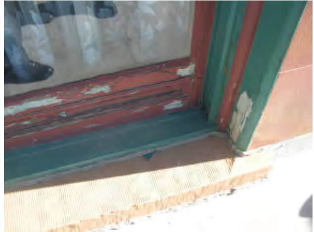
Figure IV-35. Peeling paint in 2010 on the south elevation prior to repainting.
