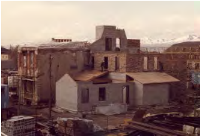
Figure III-16. A construction period photograph from the northeast showing the reconstructed laundry addition in the foreground
