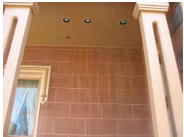
Figure IV-11. Water stains underneath the porch roof on the east elevation.
