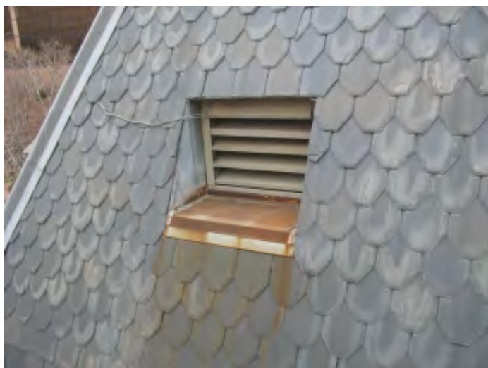
Figure IV-29. A mechanical room air duct penetrating the slate roof on the east wing.
