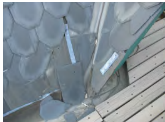
Figure IV-21. Slate repairs using a lead strip which has failed to hold the repair slate in position.
