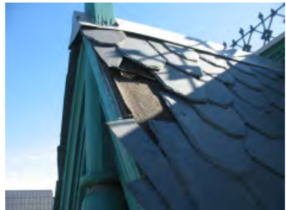
Figure IV-20. An area of missing slate showing the building paper and plywood underneath.
