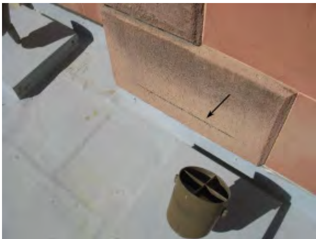
Figure IV-10. An EIFS quoin with a horizontal crack which allows water to enter the wall system.
