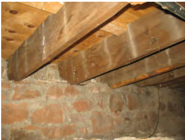
Figure III-28. A detail of the floor joists under the Drawing Room supported by a shelf in the foundation wall.
