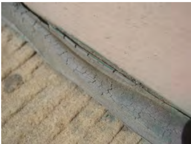
Figure IV-14 (below left). A detail of a failed sealant bead at the junction of a sandstone sill and the wall.
