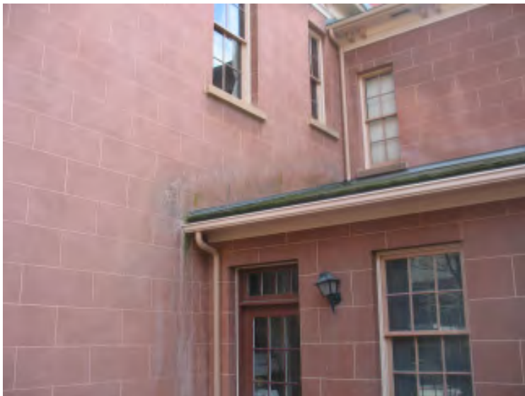
Figure IV-34. A view of the lower kitchen roof showing water staining on adjacent stucco walls.
