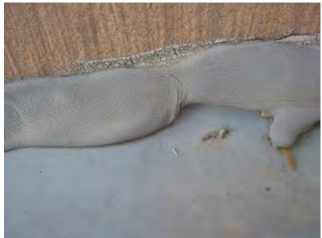
Figure IV-15 (below). A detail of newer sealant installed over older sealant.
