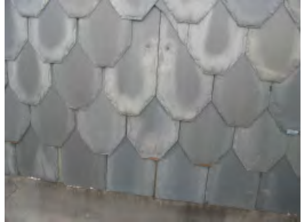
Figure IV-22. A detail of slates repaired with copper and lead tabs. Note the missing slate in the center of the photograph.
