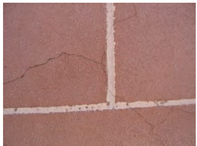
Figure IV-4. A close-up of the stucco surface showing the painted joint lines and cracks.
