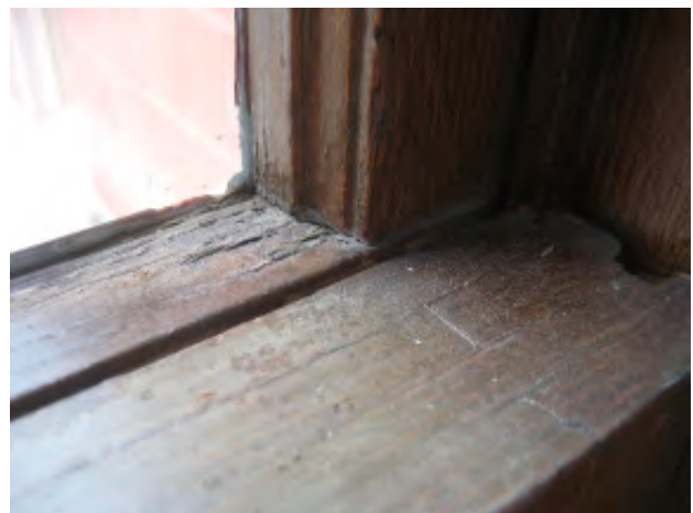
Figure IV-37 (below). A detail showing a deteriorated window sash where condensation pools at the bottom rail.
