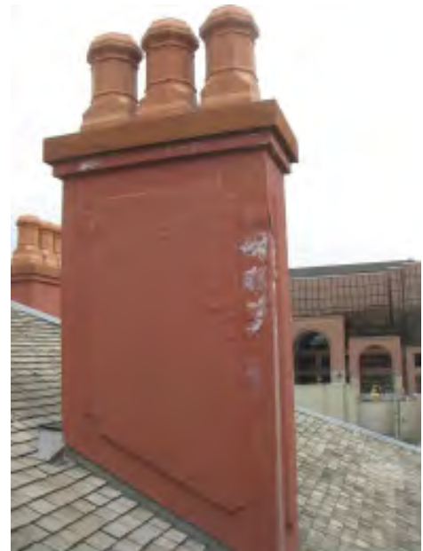
Figure IV-8 (top). A chimney with a bubbled elastomeric coating and efflorescence staining the surface.
