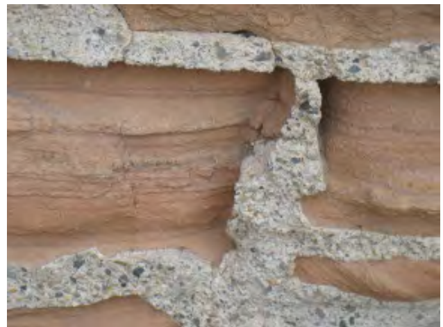
Figure IV-2. A detail of the west foundation wall showing the eroded sandstone around the hard mortar.
