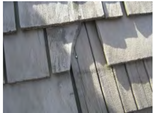
Figure IV-31. A split shingle which has exposed the nail of the shingle underneath.
