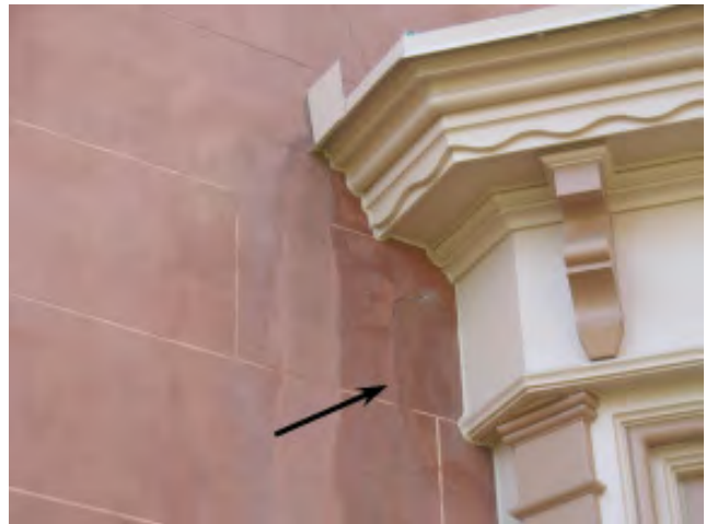
Figure IV-6. A detail of the cracks at the location of the lintel bearing at the Dining Room east bay window.
