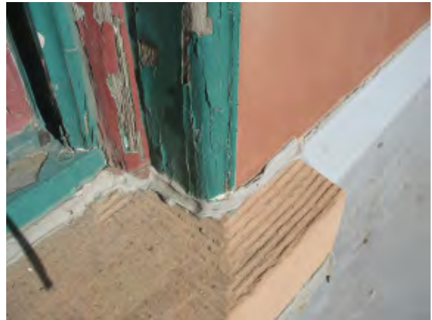
Figure IV-36. Peeling paint in 2010 on the south elevation.
