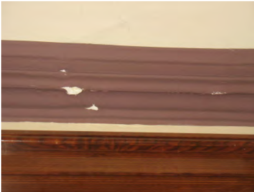
Figure IV-18. Water damage on a plaster crown molding in the Entrance Vestibule.
