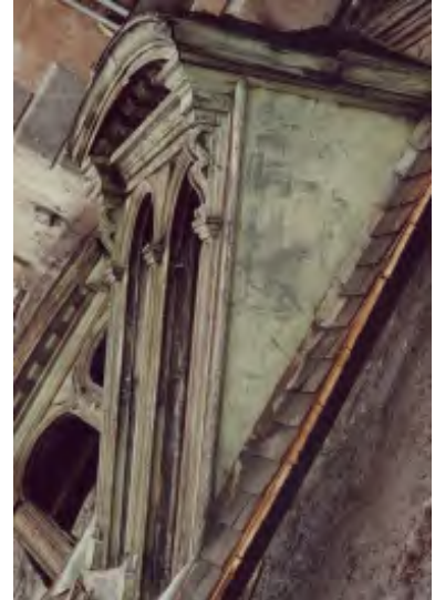
Figure III-6 (right). An original dormer cut from the roof and resting on the ground during restoration (the photograph has been rotated for clarity).
