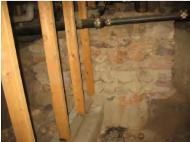
Figure III-30. The foundation of the original kitchen fireplace in the west wing, and a new support wall bearing on a concrete footer.
