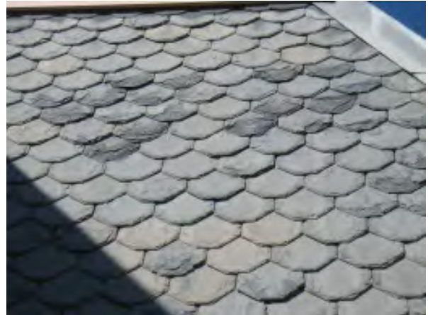
Figure IV-19. A detail of weathered slates on the south elevation.
