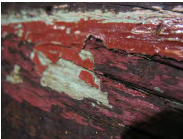
Figure V-7. The weathered surface of a painted board originally part of a panel on the bottom sash of a window.
