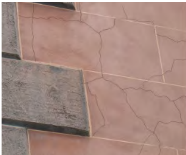
Figure IV-3. A detail of the stucco surface and quoins showing the cracking pattern on the stucco surface. Cracks have been outlined for clarity.
