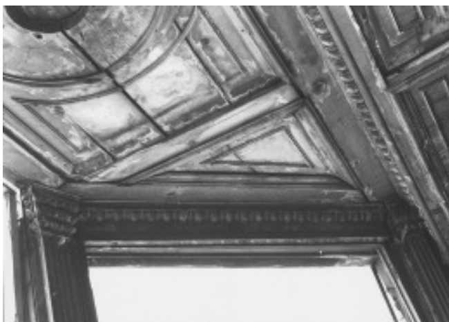
Figure III-38. A view of the projecting bay soffit before restoration, HABS #U-37, photo #19.
