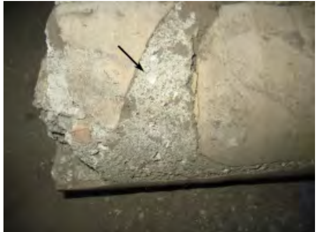
Figure III-27. A view of a 5 inch core of the foundation wall showing white lumps of lime in the mortar.
