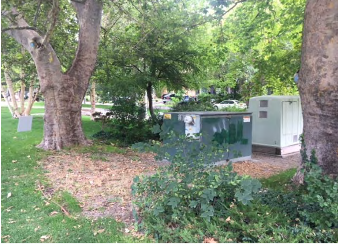
North/Eastern View of Existing Well
