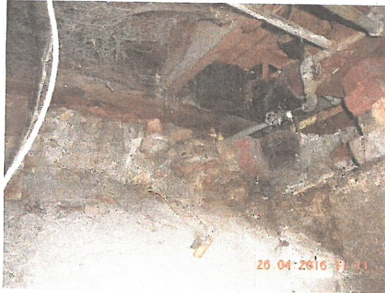
Photo 5 – Inadequate load transfer connection at deteriorating foundation
