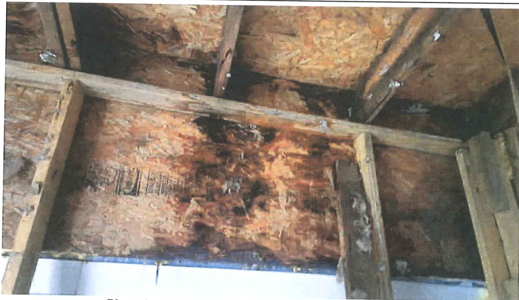
Photo 2: Water damage from improper roof drainage
