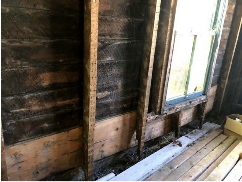
Image 1 - Existing North exterior wall being pushed by the current grading to be reinforced with new exterior retaining wall and foundation wall.
