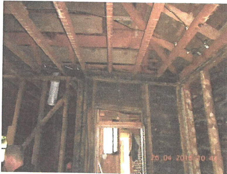
Photo 72 – Apparent settlement at west wall
