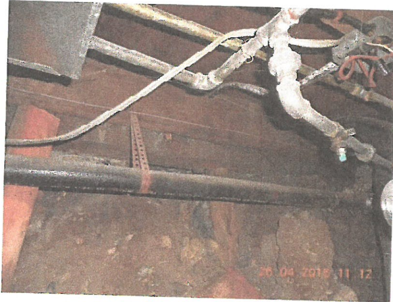
Photo 7 – Inadequate load transfer connection at deteriorating foundation
