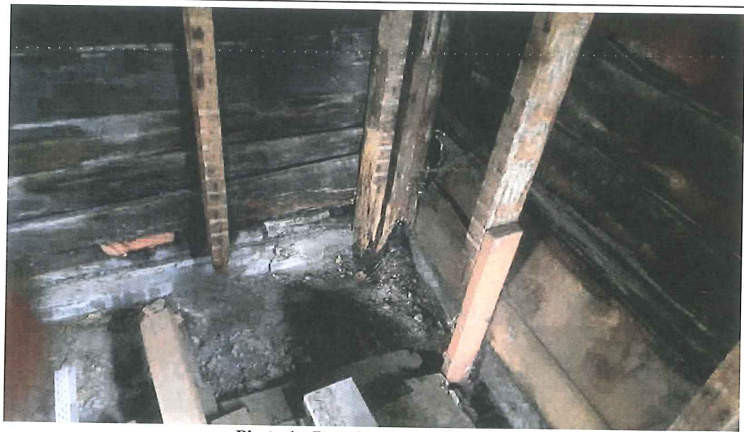
Photo 1: Deteriorated walls studs
