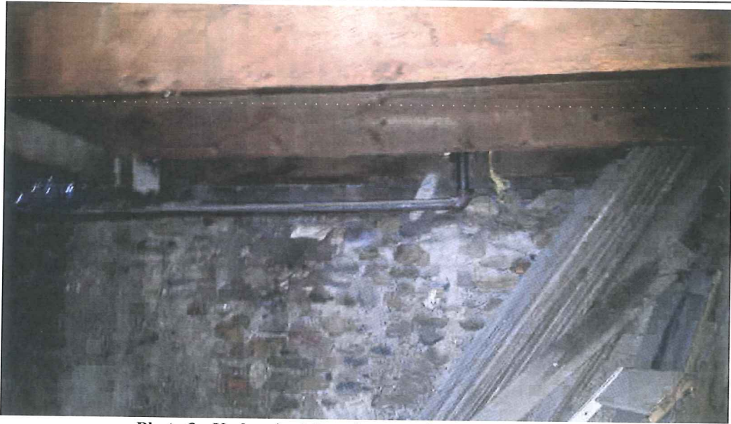
Photo 3: Under sized floor beam and cobble foundations.
