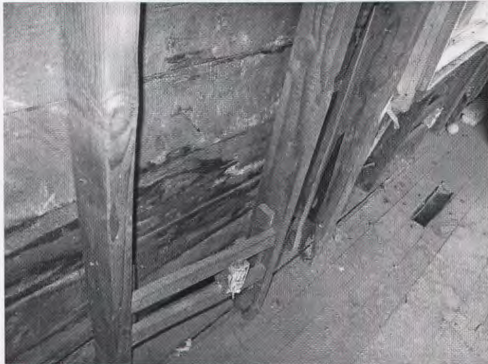
Examples of structural deficiencies.
