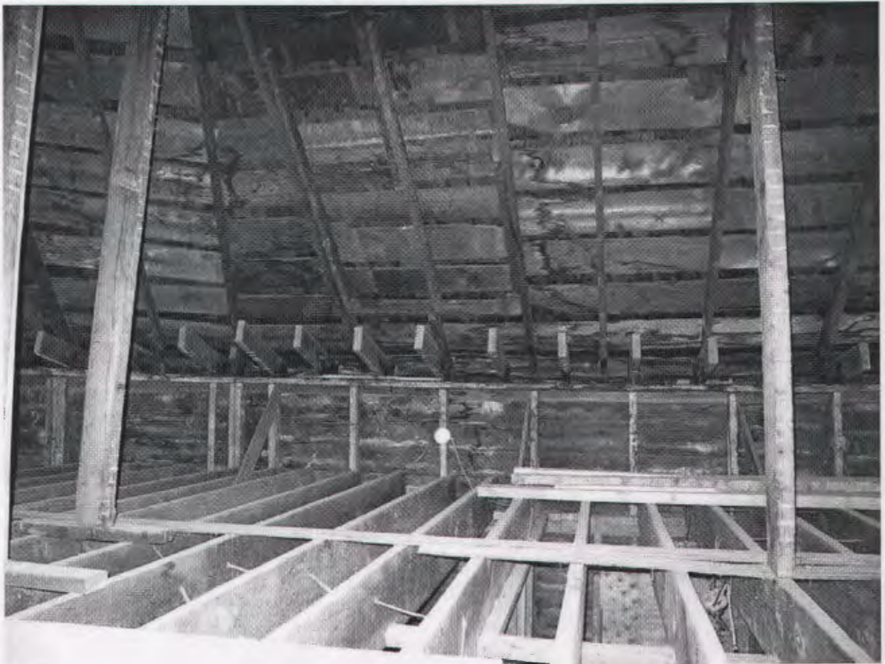
The lower roof cords have been cut, with the remaining pieces rising up as the roof settles.
