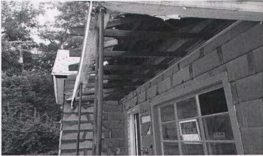
Photo 11: Deteriorated front porch beam
