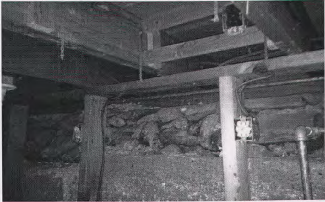
Photo 9: Concrete foundation walls to the interior of original stone and mortar walls
