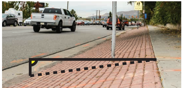
Foothill Drive has a number of narrow sidewalks with significant park strip slopes toward the street which present safety hazards for pedestrians and users with disabilities.
