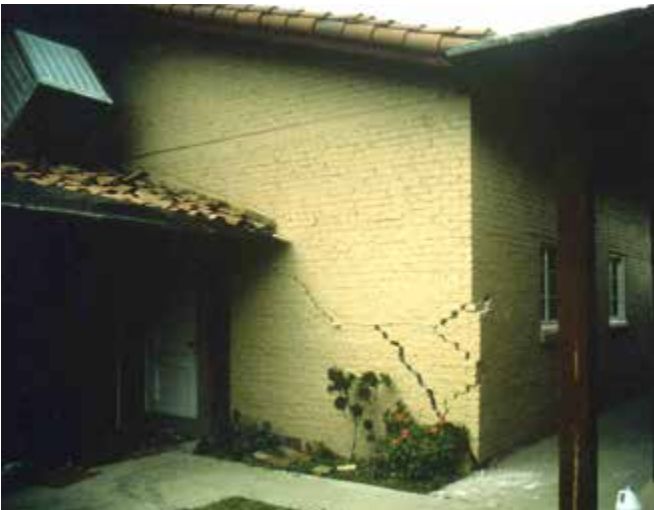
Figure 7. Earthquake damage to an URM wall and displacement of mechanical equipment on roof.
