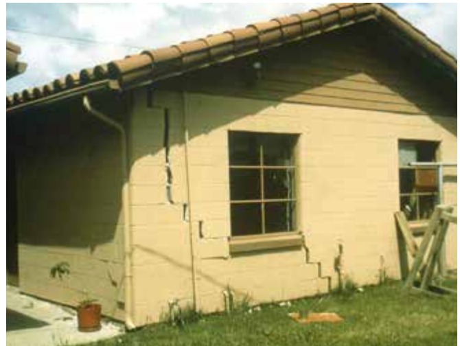
Figure 8. URM wall failure from an earthquake.
