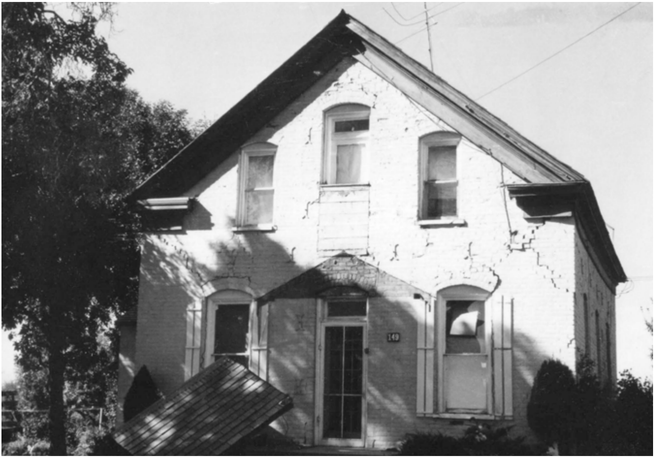
Figure 2. Cracks and failure due to an earthquake. Photo: Ariel Benson.
