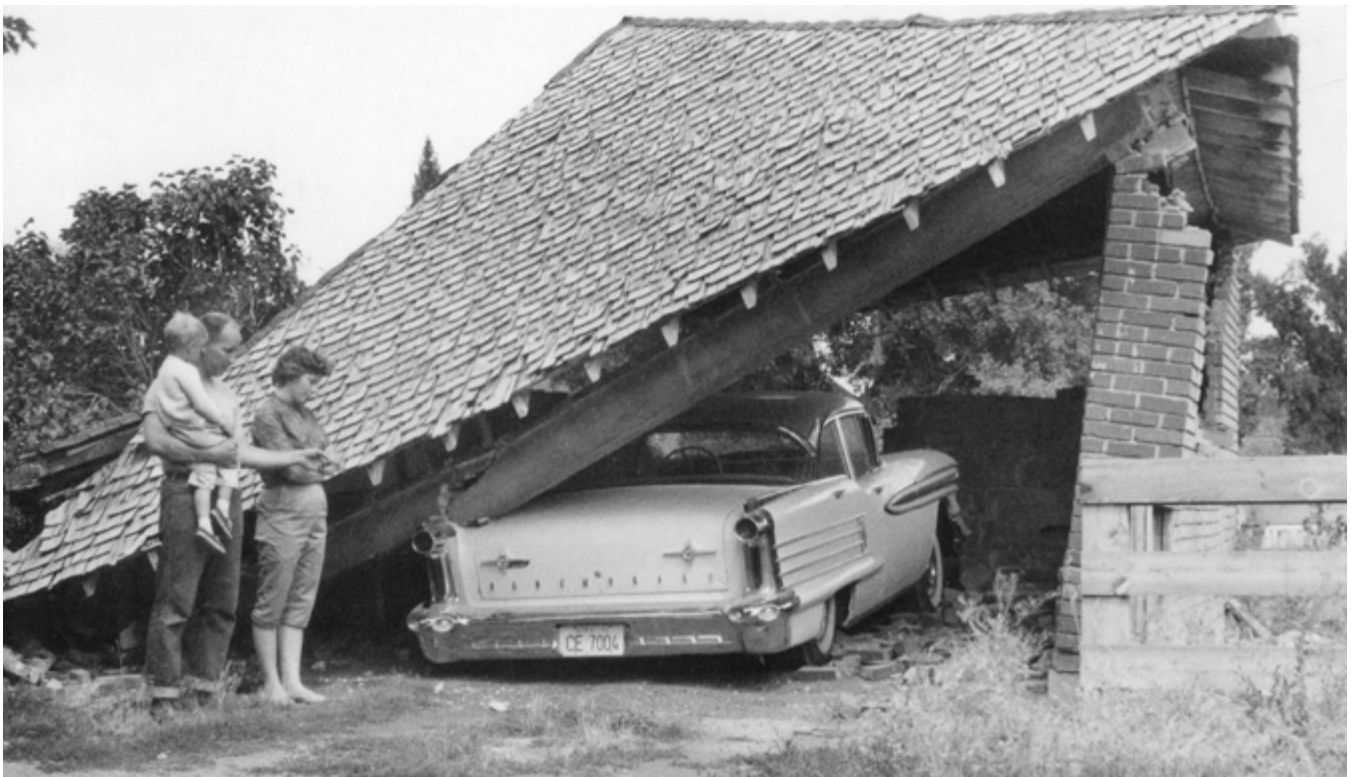
Figure 9. URM pier failure. Photo: Ariel Benson
