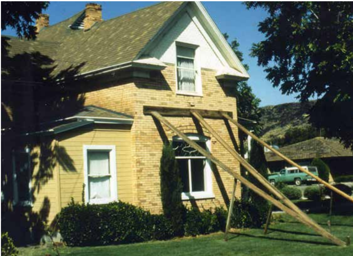
Figure 1. Braced exterior wall of a URM dwelling after an earthquake.
