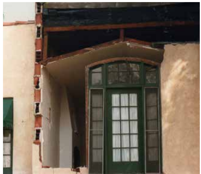
Figure 5. URM wall (hollow clay units) collapse due to earthquake.
