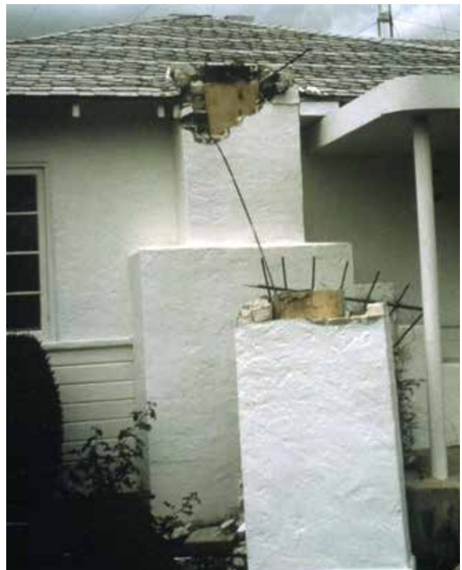
Figure 11. Chimney failure due to inadequate reinforcement.
