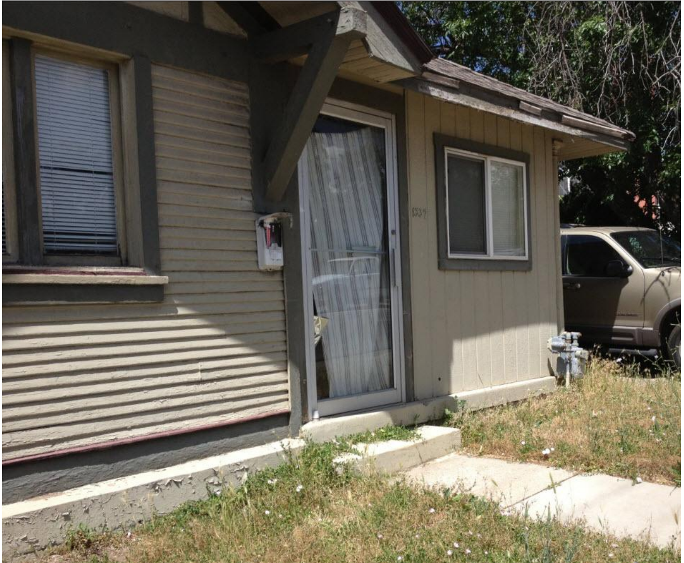
Close up of eastern portion of the five panel window and siding, 2013
