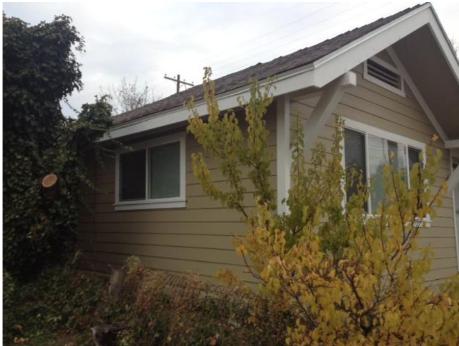
West façade after modifications (The only vinyl replacement window staff recommends approval of is hidden behind the tree in the photo)
