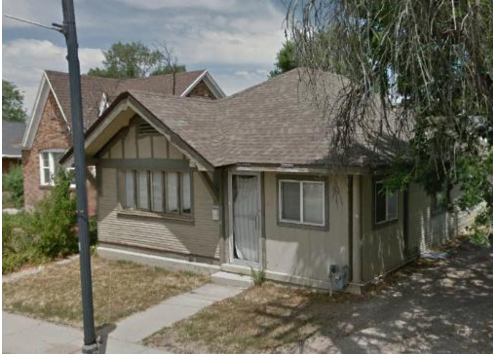
Photo of the historic cladding, the detailed eave and the Corinthian column prior to modifications
