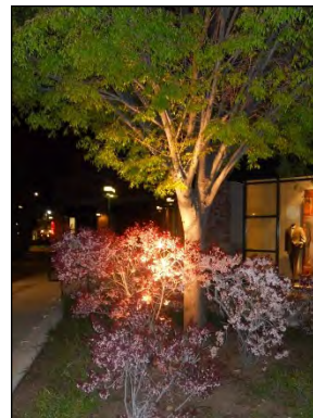
Landscape lighting can be used to highlight unique landscape features and help improve the safety of public spaces.
