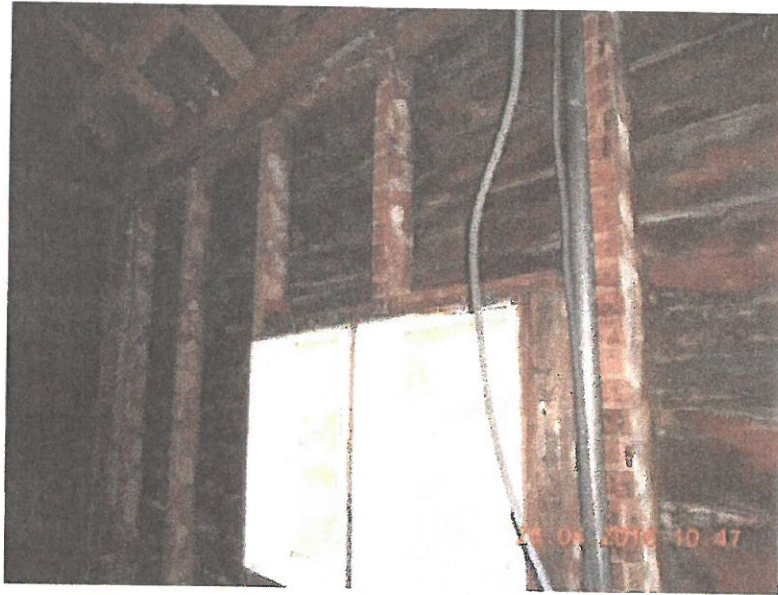
Photo 61 – No headers, king studs at wall openings
