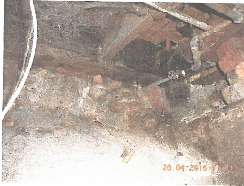
Photo 5 – Inadequate load transfer connection at deteriorating foundation
