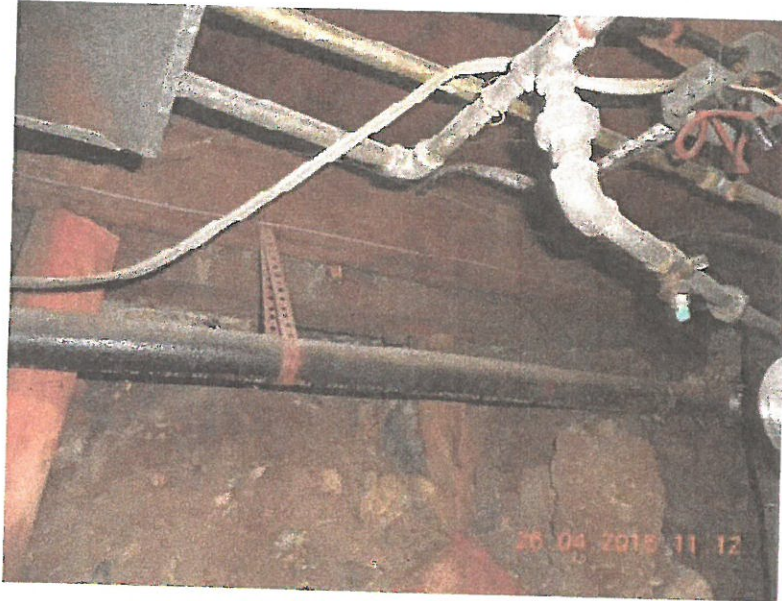
Photo 7 – Inadequate load transfer connection at deteriorating foundation
