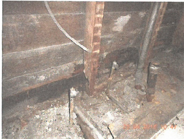
Photo 10 – Deteriorated foundation, sill plate, studs, and floor joists
