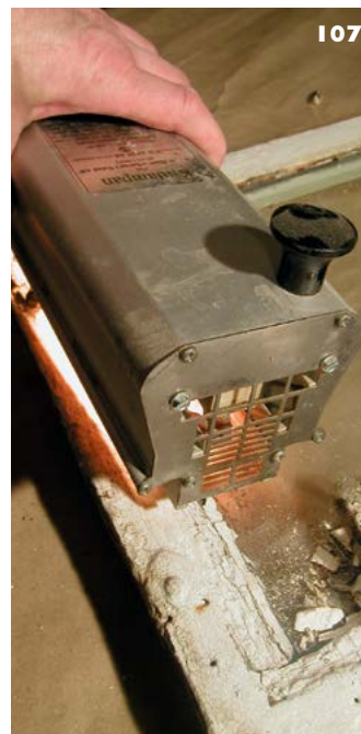
106: Steel window showing severe corrosion to the bottom rail of the frame and distortion from 'rust jacking' which has cracked the glass.
