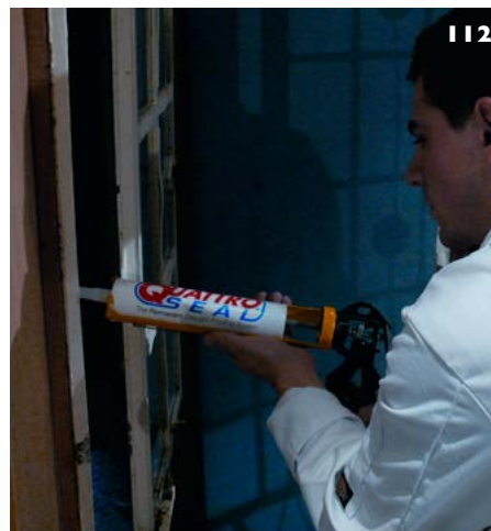
112: Silicone being injected into gaps between the frame and casement to exclude draughts. The casement is first painted with a releasing agent. The silicone is then left to cure with any excess trimmed back.
