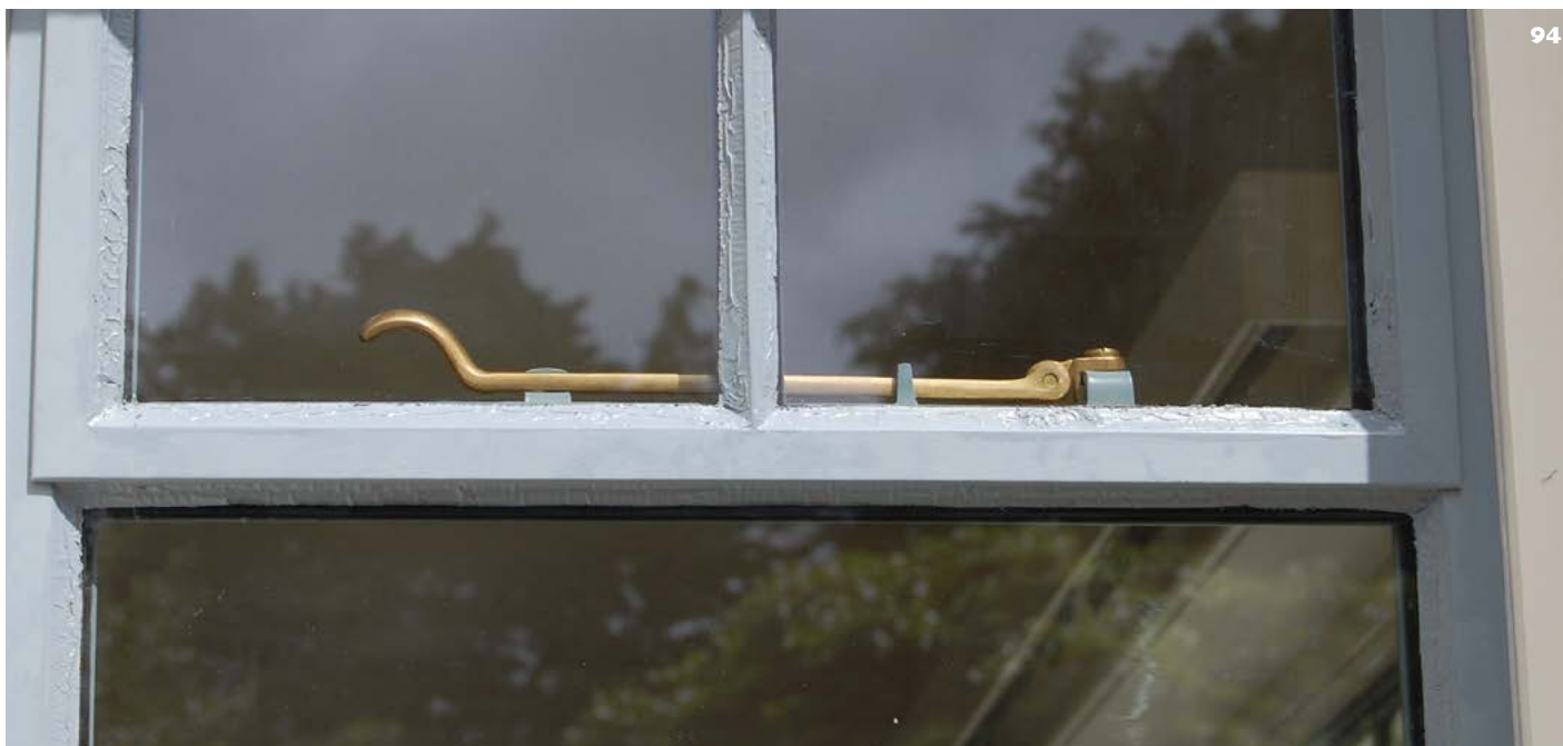
94: The new putty to this steel casement hasn't been allowed sufficient time to cure before being painted. Consequently the paint has blistered.
