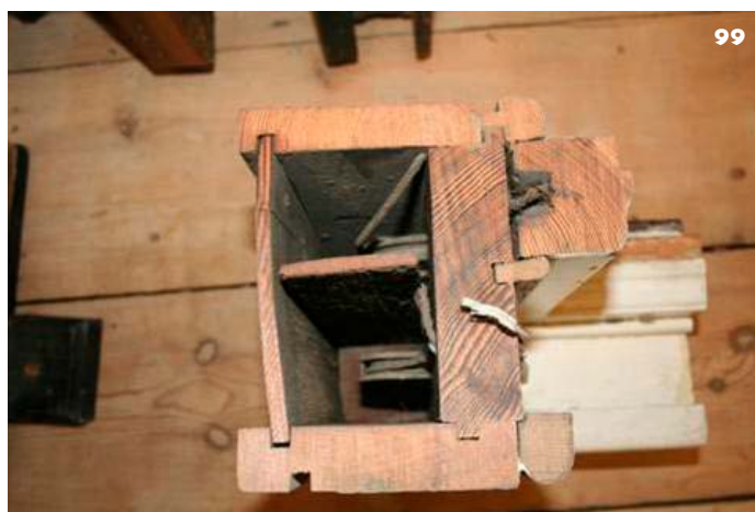
99: This section through a sash box shows the high quality of the timber used during the 19th century.
