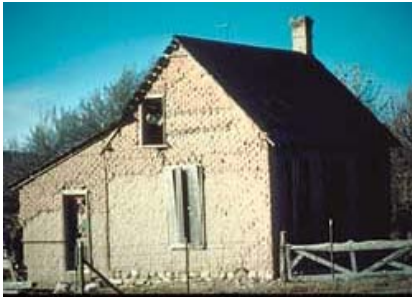
A traditional mixture of mud and straw plaster should be applied to stabilize the exterior of this house. Photo: NPS files.
