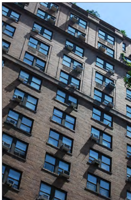
Retrofitting equipment individually can have a significant visual impact on an older building.
