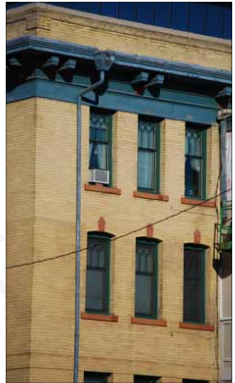
Classical window proportion and detail, and solid to void ratio, establish a very distinct sense of human scale.
