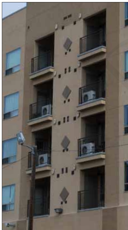
Retrofitting AC equipment on a new building is an issue that should not arise.
