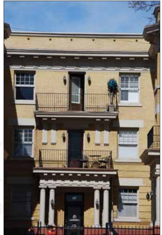
Window reveals and frame detailing designed as part of the facade composition.
