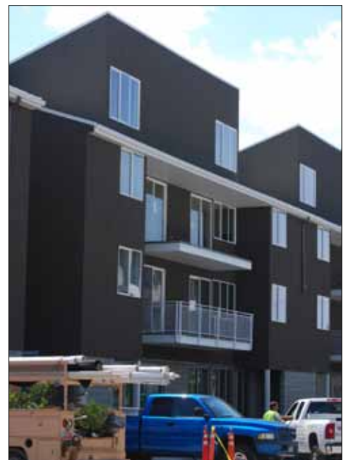
Broken massing and projecting balcony space create a repeating facade module of limited interest or durability.
