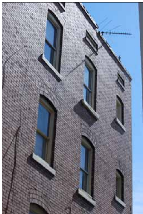
Reading the texture of a brick wall conveys a sense of permanence, durability and construction, as well as the detail provided by the patterns of coursed and arched brickwork and projecting sills.
