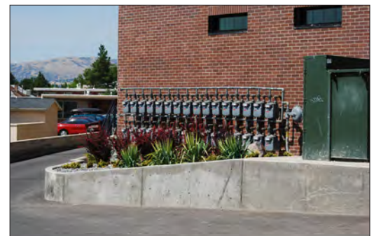
Screening of utility service meters in this instance will rely on maturing landscaping and subsequent maintenance.
