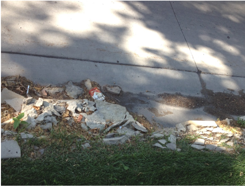
Damaged limestone curb
