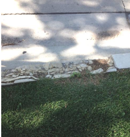
Failing Limestone Curb
