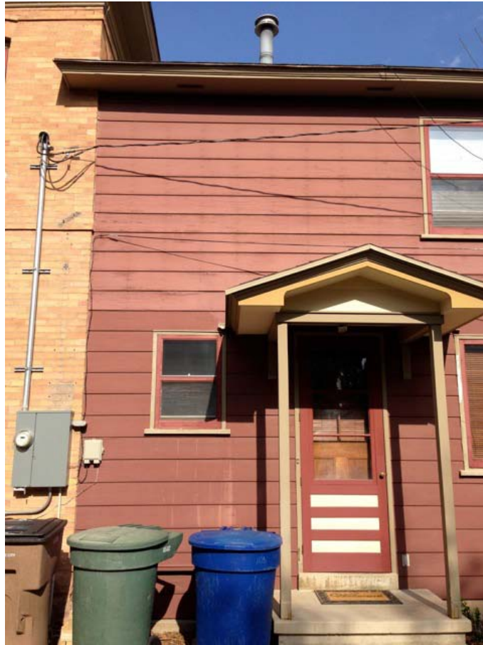
Covered entryway will remain – the existing porch columns will replace these ‘stick’ columns
