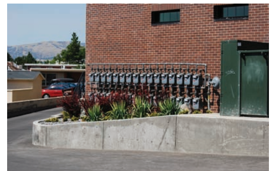
Screening of utility service meters in this case will rely on landscape maturity and subsequent maintenance.
