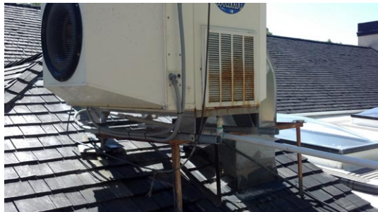
5-ton Coolerado unit for Garden Room
