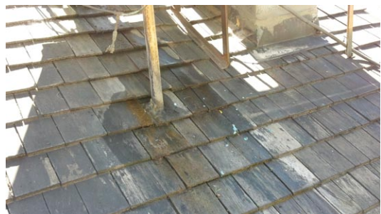
Leak from 5-ton Coolerado unit for Garden Room onto wood shingle roof
