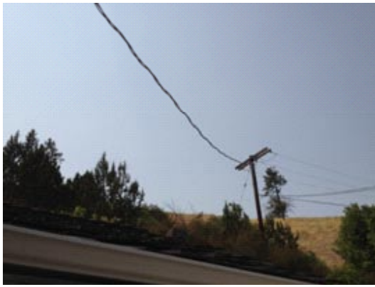
Power pole feeding building
