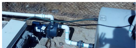
Pump and tank to pump waste water from Coolerado units to irrigation system
