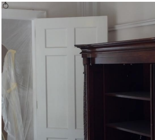
Thermostat for Main Hall in Corridor hidden behind the open door to the Main Hall
