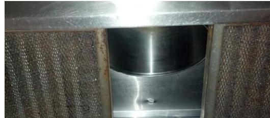
Kitchen hood showing open space between filters
