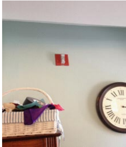
Fire alarm strobe in acceptable condition.
