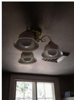
Second Floor Office Incandenscent Luminaire.
