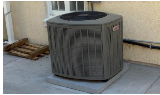
5-ton condensing unit for Main Hall
