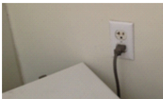
Receptacles in acceptable condition.
