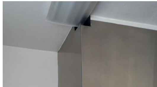
Kitchen hood showing hole for lighting fixture
