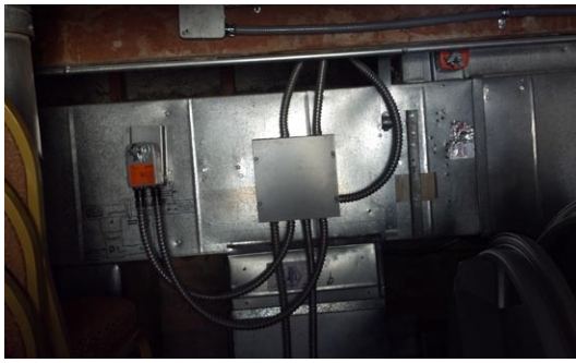
Dampers for Garden Room Coolerado unit and furnace
