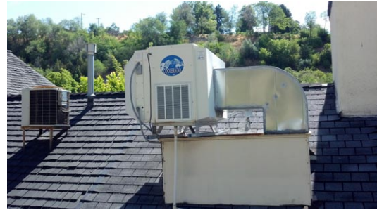
5-ton Coolerado unit for Main Hall and 2.5-ton condensing unit for second floor unit
