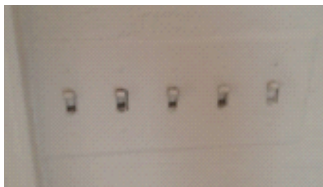
Light switches in poor condition.
