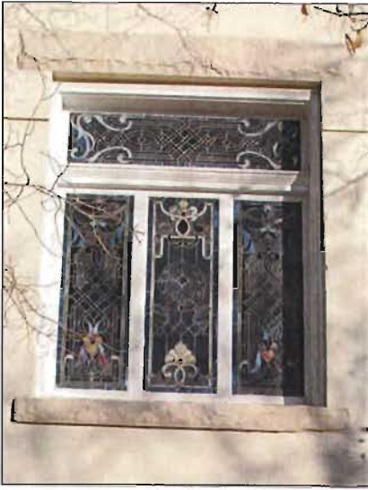
Ornamental windows such as this oval window and the stained glass window above are character-defining features that often indicate the architectural style of a house.
