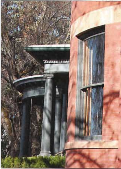
The curved sash glass and frame in these windows are distinctive features that should be preserved.
