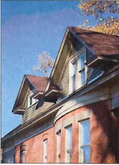
Rear addition with second story space above designed to complement and be distinguished from the original house.
