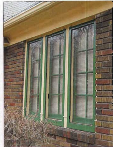
External wood framed storm windows designed to fit the primary framework of the original.
