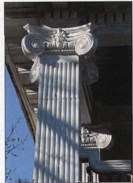
Periodic maintenance of painted surfaces maintains weather resistance and enhances the character of the building.
