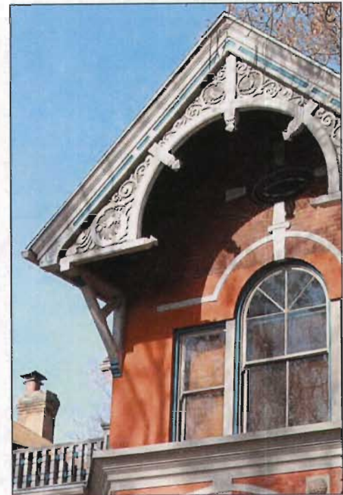
Using non-paintable substitute materials may preclude enhancing architectural details through a carefully considered color scheme.
