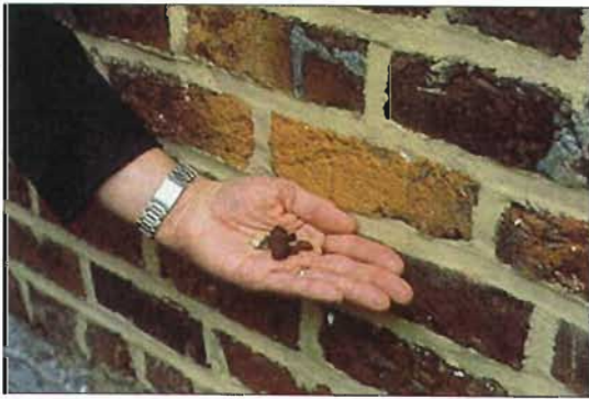
Hard impermeable modern mortars force moisture through the then more permeable brick and force mechanical stresses to be relieved through the softer brick which may lead to cracking, spalling and erosion. Here, new mortar fails to match the original.
