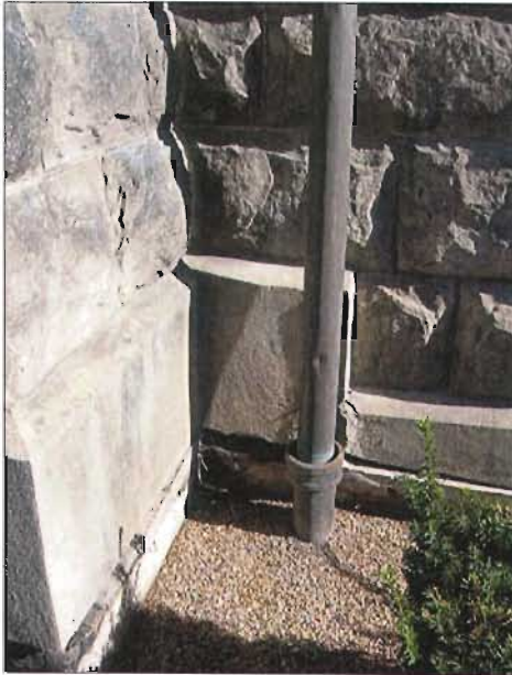
Underground downspout extensions move water away from the foundation.
