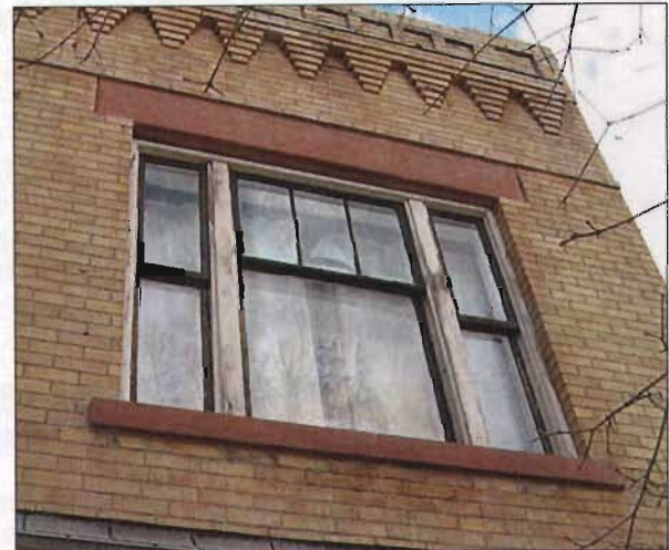
The wood framing distinguishes this historic window design, profile and detailing in an upper story window treatment.
