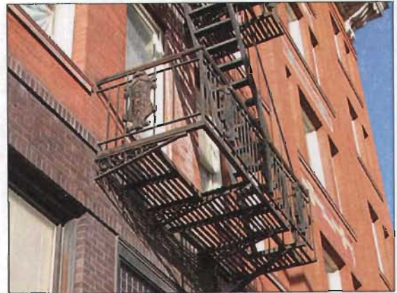
Historic fire escapes, such as the one at 379 S. Main Street, can be decorative as well as functional.
