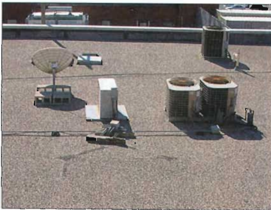
This low-profile mechanical equipment is situated in an inconspicuous area on top of the building.
