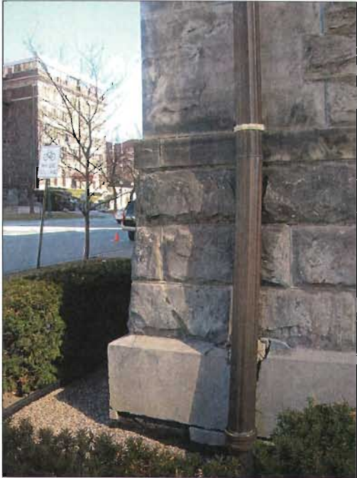
Moisture, wind-borne grit and pollutants can affect all types of foundation materials.
