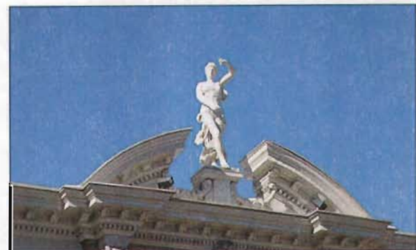
Decorative elements such as this statue at the Promised Valley Theatre are part of a building's unique roof profile.
