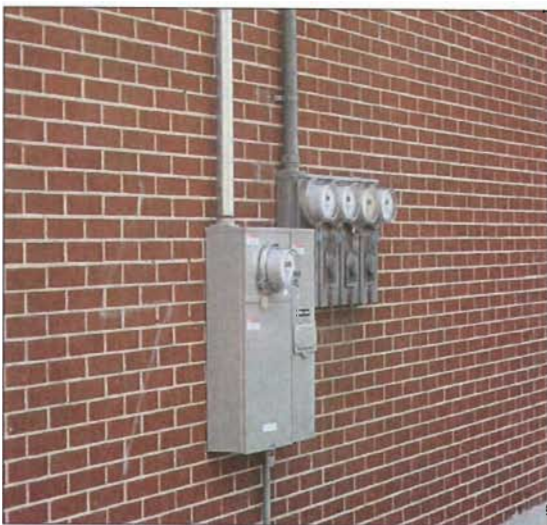
Meters are correctly placed on a non-primary facade.
