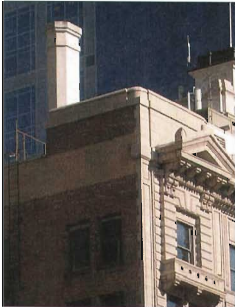
A decorative chimney can be a unique element of the city's skyline.
