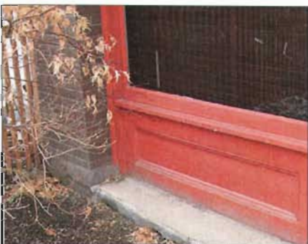
Original wood bulkheads such as those at 361 N. Main Street are central elements of historic storefronts.
