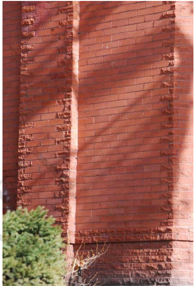
Brickwork, including the bond and mortar joint width and profile, may be an essential component of the architectural character
