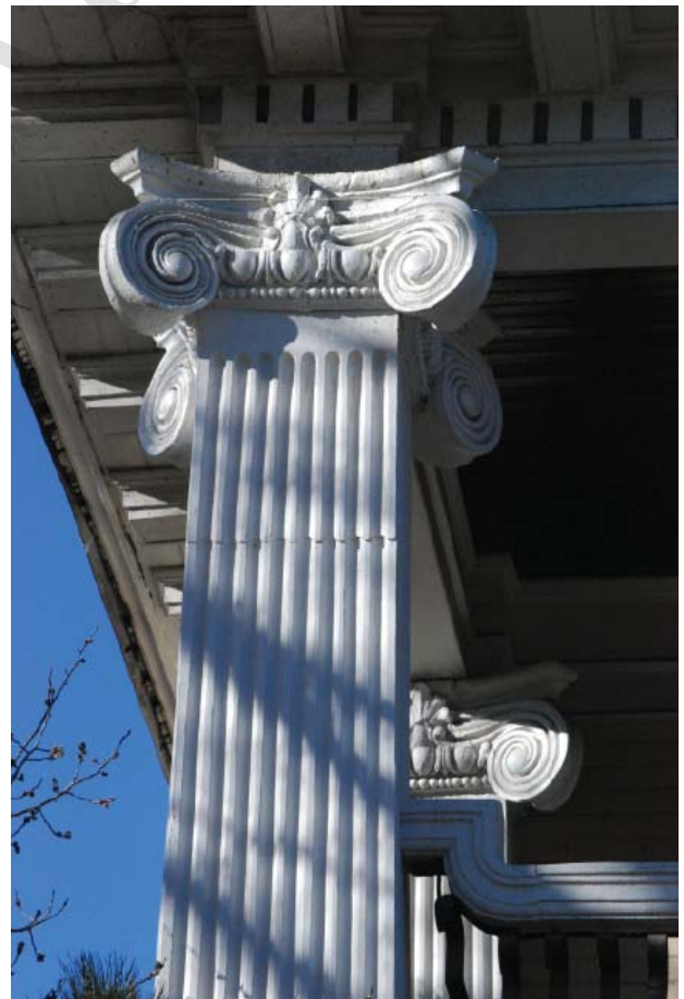
Periodic maintenance of painted surfaces maintains weather resistance and enhances the character of the building.
