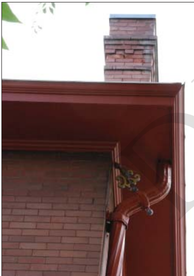
Gutters and downspouts may be a considered part of the building design.
