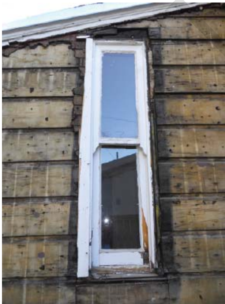
Removing later materials should reveal the original materials, which with care can be successfully repaired
