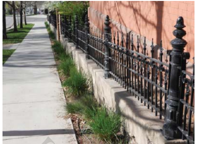
The low retaining wall supporting an ornate historic iron fence contributes significantly to the character of the streetscape.
