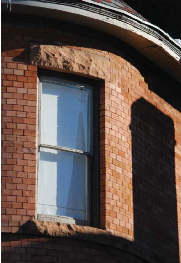
The appearance and integrity of the original masonry can be successfully maintained through appropriate repair.
