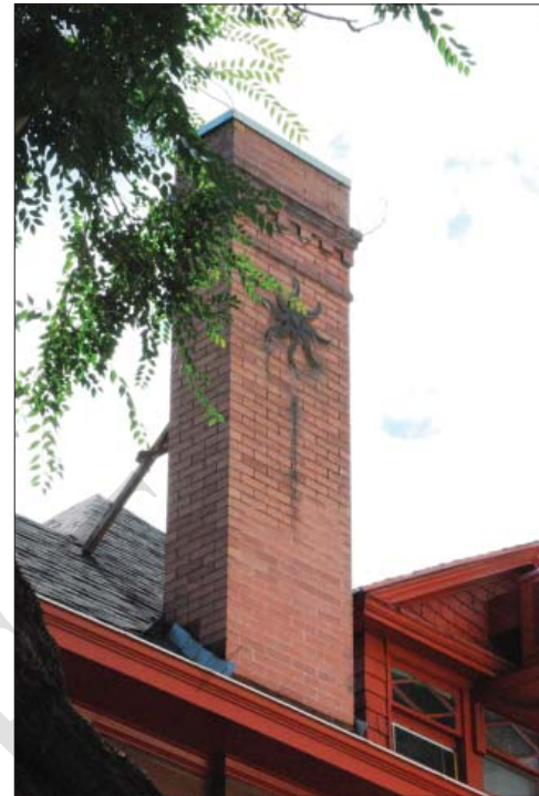
Seismic bracing on one of the many decorative chimney stacks in the city.
