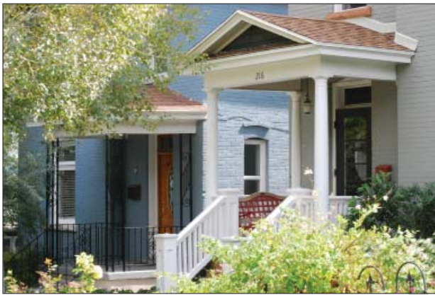
Wood columns and balustrades were commonly replaced with thin "wrought iron" railings and posts in the 1950s. This compromised the proportions and architectural integrity of the house.
