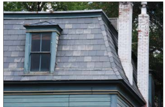
Natural slate is rare in the city and is the most durable of traditional roof materials, usually requiring
