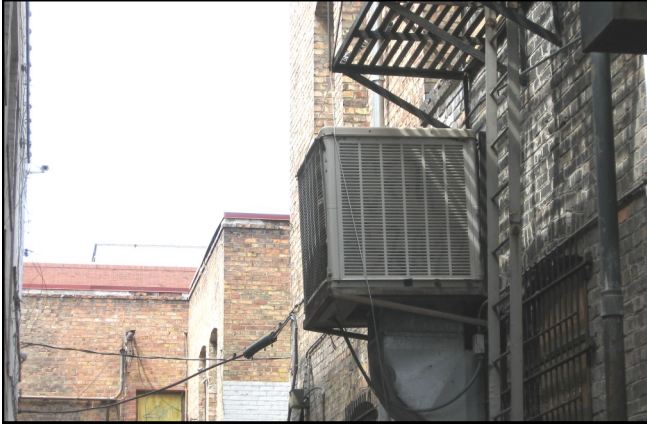
Heating and cooling units should be located at rear elevations such as shown here or on rooftop areas not visible from the street.
