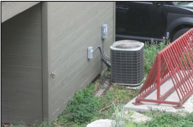
This HVAC system at 271 N Center Street is situated in an inconspicuous area on the rear elevation.
