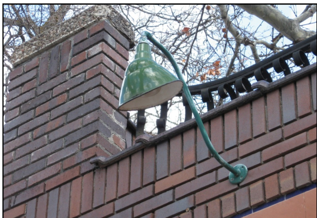
Swan- or goose-neck fixtures in dark metals are appropriate new light fixtures for commercial buildings, as at 82 N 'Q' Street (left) and 422-426 N 300 West (right).
