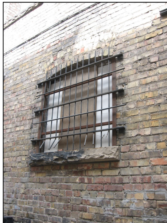
Security bars are more appropriate on side or rear elevations.
