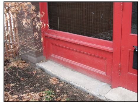
Original wood bulkheads such as those at 361 N Main Street are significant parts of historic storefronts.
