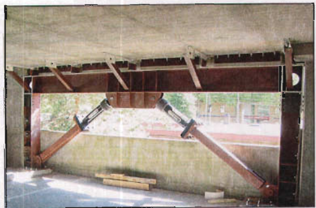
Seismic retrofitting can include adding steel frames and dampers in basement and parking areas of commercial buildings.
