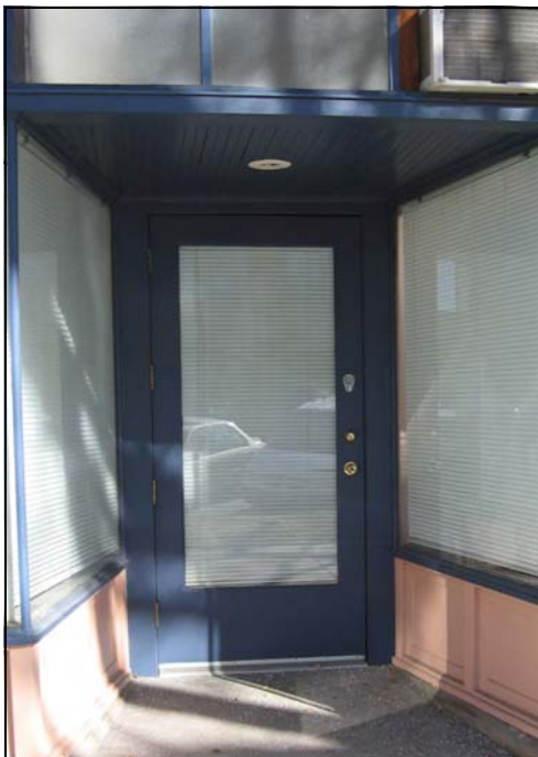
Rebuilt doors, such as this example at 428 W 300 South, replicate the original as closely as possible.
