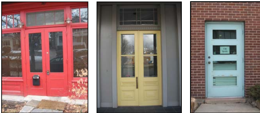
Salt Lake City’s commercial buildings have a variety of doors and entrances: Original double doors at 361 N Main Street (left) and 740 E 2nd Avenue (center), and an original steel door at 736 N 300 West (right).
