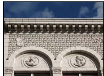
Architectural details exhibit craftsmanship and help convey a building's distinct character. Above: Felt Building, 341 S Main Street.
