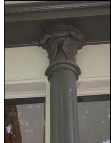
Cast iron details add to the historic character of a building (68 N 'K' Street).
