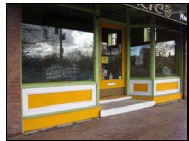
Preserve and maintain original storefronts, such as those at 802 S 600 East (top) and 779 S 500 East (bottom).
