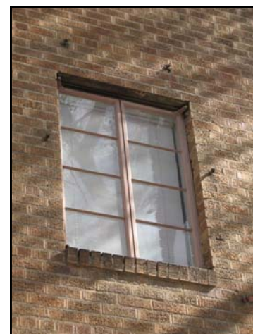
Original steel casement window at 702 N 'K' Street. This window is significant to the design and character of the building.
