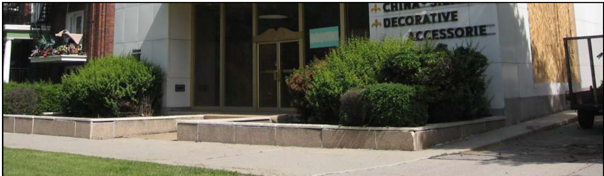
Preserve and maintain masonry retaining walls in front of commercial buildings such as this example at 445 E South Temple Street.
