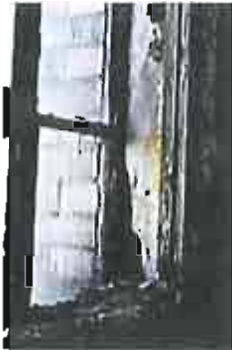
The extensive deterioration of this historic metal window justifies its replacement with a matching new window. Photo: NPS files
