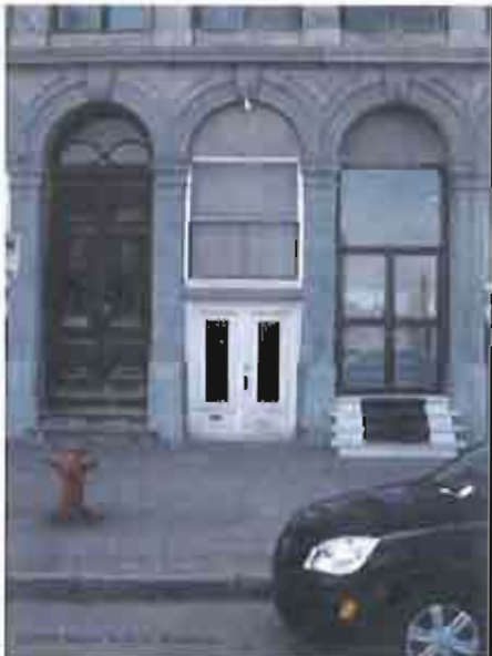
Windows are not the only elements maligned by inappropriate replacements.
