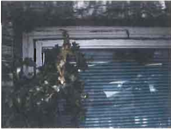
Replacing sash while ignoring the primary sources of infiltration can have detrimental and costly results.
