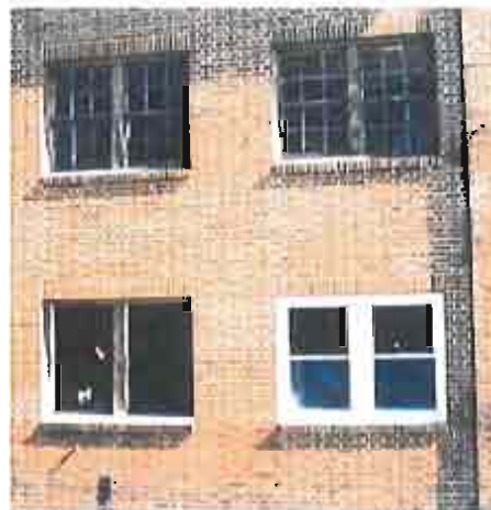
Incompatible new window (lower right), resulting in loss of the building's historic character.
