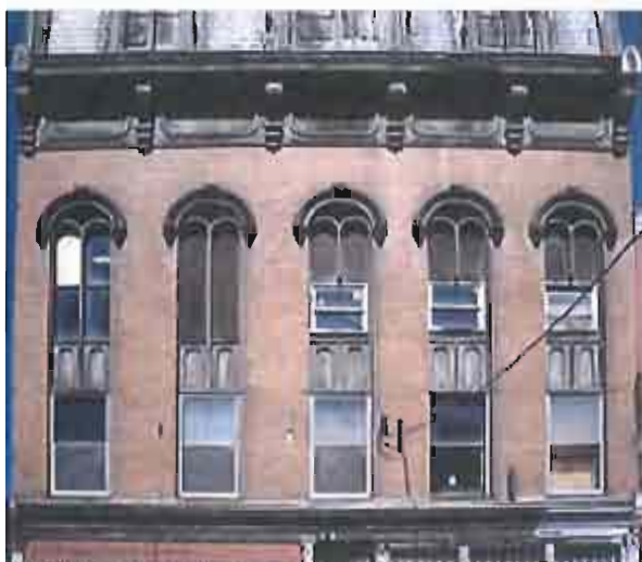
The damage wrought by replacement windows is self-evident and increasingly pervasive. All photos: © Walter Sedovic Associates
