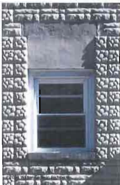
This window replacement resulted in reduced visibility and daylight.
