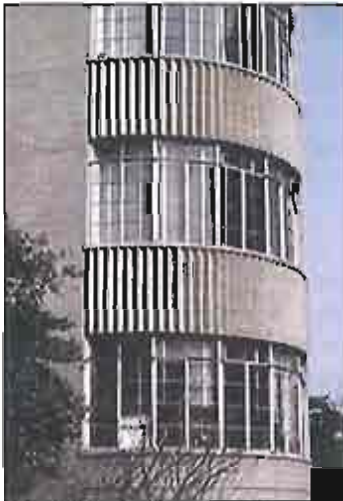
The historic steel sash is shown in place, prior to its removal and replacement with inappropriate aluminum sash (see below). Photo: NPS files.
