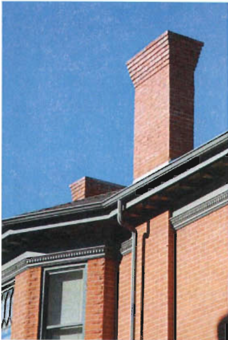
Variation in the brick texture and the pointing profile are used in this case to define the wall, the window bay and the chimneys.
