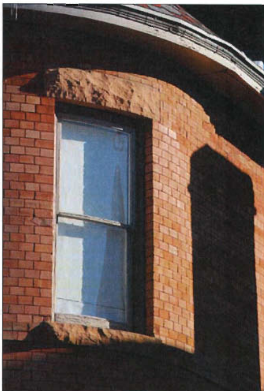
The appearance and integrity of the original masonry can be successfully maintained through appropriate repair.
