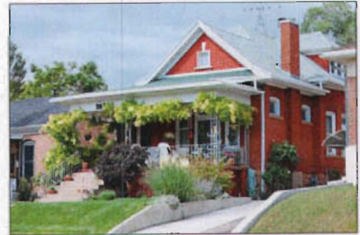
This porch has been altered and, as a result, the historic character is compromised.
