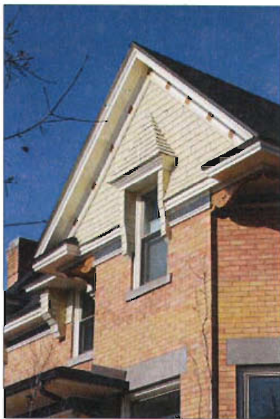
Original materials are essential to the integrity of a building and convey a sense of authenticity and maturity.
