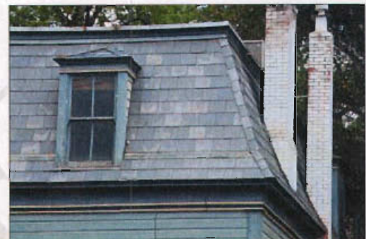
Natural slate is rare in the city and is the most durable of traditional roof materials, usually requiring only piecemeal replacement of damaged individual slates.
