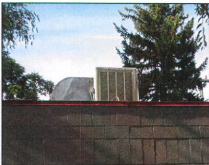
This roof mechanical system is set back so that it is not readily visible from the street.
