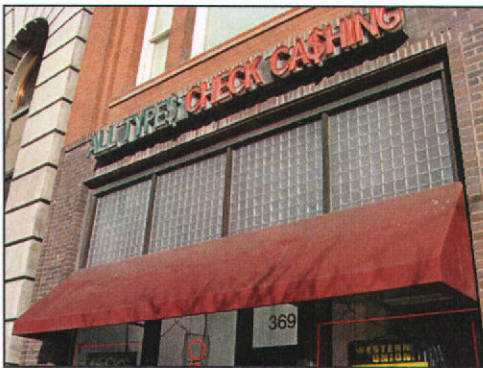
The distinctive Luxfer glass transom on the New Grand Hotel at 369-379 S Main Street is intact and not concealed.
