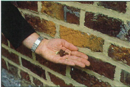
Hard impermeable modern mortars may force moisture through the more permeable brick and force mechanical stresses to be relieved through the softer brick...which may lead to cracking, spalling, and erosion.
