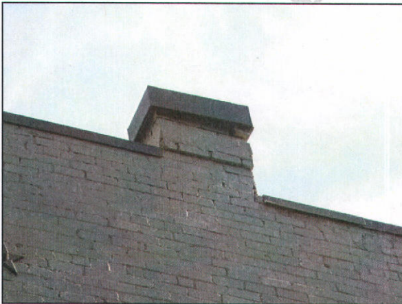
This chimney is incorporated into the building façade at 68 N 'K' Street.
