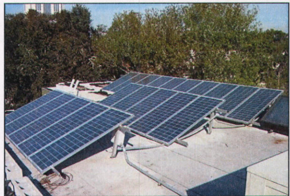
Rooftops are an appropriate location for solar panels.
