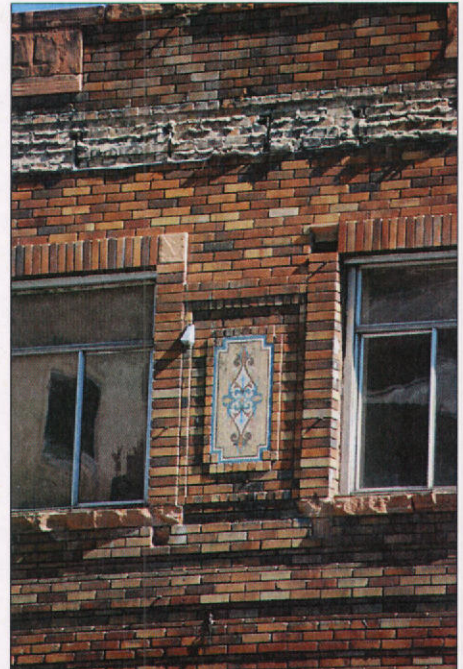
Provide proper drainage so that water does not stand on flat, horizontal surfaces.
