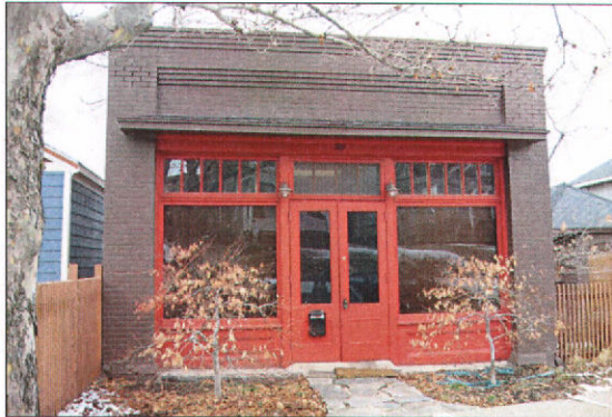
Woodwork is a character-defining feature of this storefront at 361 N Main Street.
