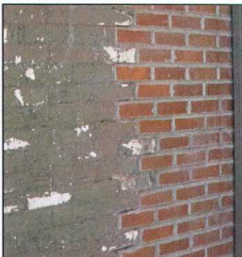
Painting brick changes the character of the building.
