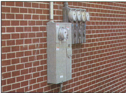
Meters at 39 N 'I' Street are correctly placed on a non-primary façade.
