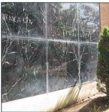
Marble paneled veneer on the main façade at 641-645 E South Temple Street.
