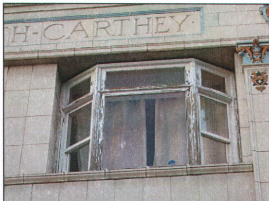
Regular maintenance will improve the longevity of a historic window.
