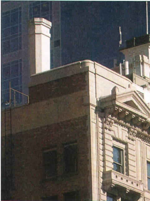
A decorative chimney can be a unique feature of a historic building's roof profile.
