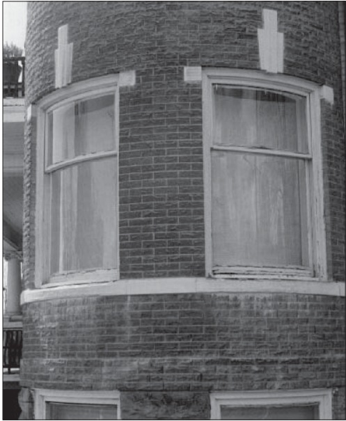
The curved sash glass and frame in these windows are distinctive features that should be preserved.
