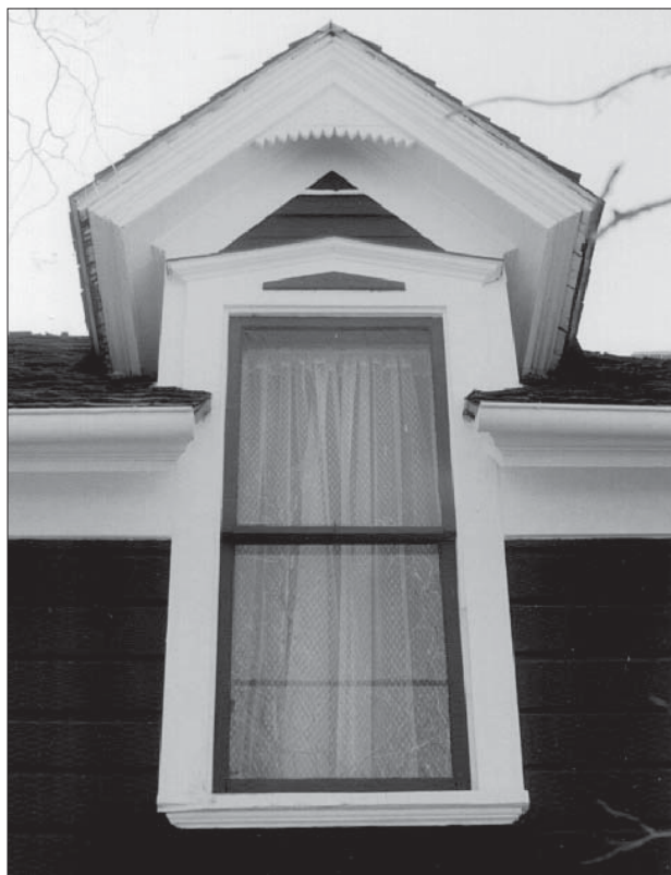
As a general rule, a window merits preservation, with perhaps selective replacement of elements, when more than 50 percent of the window components can't be repaired.
