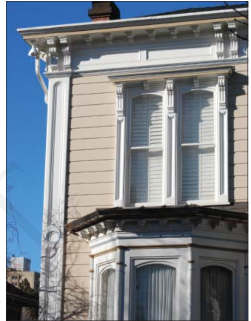
Preserving original architectural details is critical to the integrity of a building and its context.
