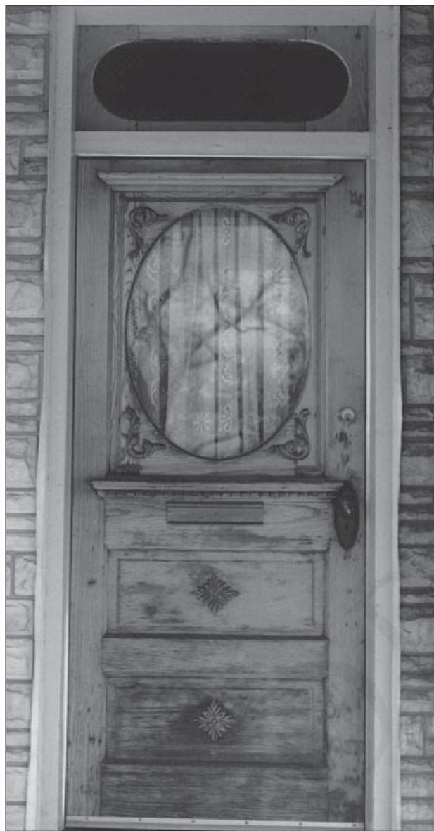
When a historic door or its components are damaged, repair them and maintain their general historic appearance.
