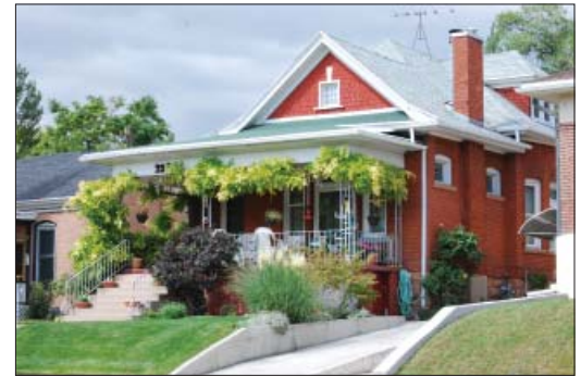
This porch has been altered and, as a result, the historic character is compromised.
