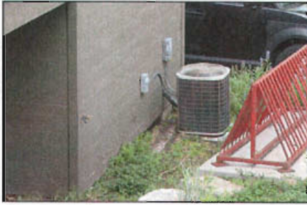
This HVAC system at 271 N Center Street is situated in an inconspicuous area at the rear of the building.
