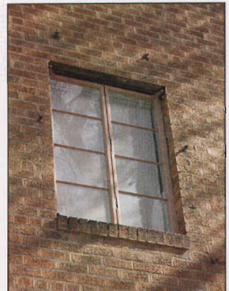
Traditional steel casement frames characteristic of certain building styles of the 20th century.
