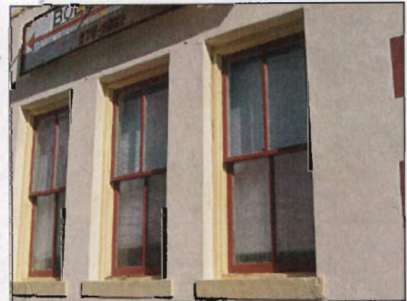
The number and position of glass panes are important to the character of a building.
