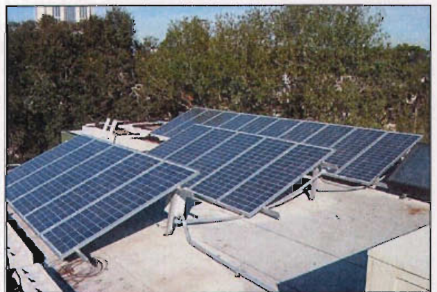
Rooftops are the preferred location for solar panels.
