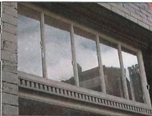
Original transoms contribute to the character of this historic storefront at 271 N Center Street.
