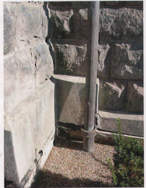
Underground downspout extensions move water away from the foundation.
