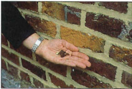
Hard impermeable modern mortars may force moisture through the more permeable brick and force mechanical stresses to be relieved through the softer brick...which may lead to cracking, spalling, and erosion.
