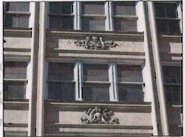
Window configuration and detailing can be important to the composition of the façade.
