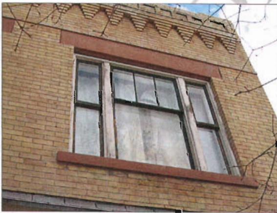
Wood framing distinguishes a historic window profile and detailing on an upper story window treatment.
