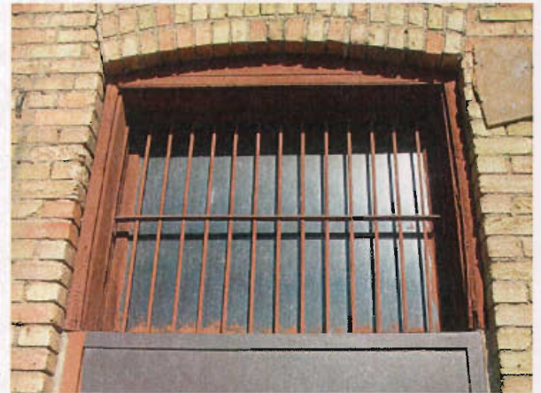
Security bars are more appropriate on side or rear elevations.
